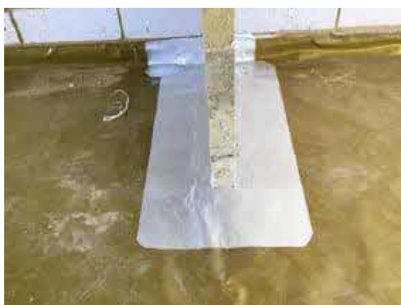
Plot 3 retro fit detail over the damaged membrane that is under the internal block work wall.
