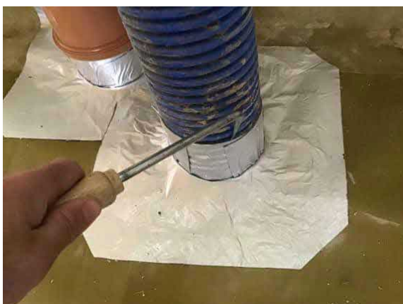
Pick testing all SAGM detailing in plot 52.
