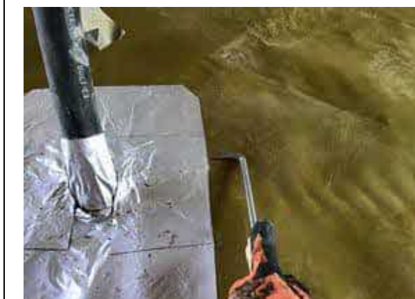
Plot 35 pick testing all SAGM detailing.
