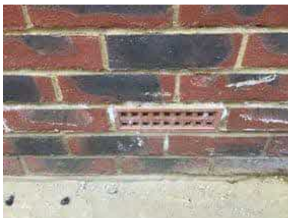
Air brick in place at the time of our inspection to plot 65.
