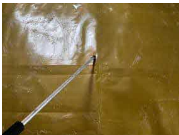
Plot 72. Air lance integrity test conducted upon hand welded lap joint.
