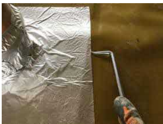
Plot 6 pick testing all SAGM detailing.
