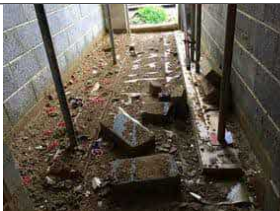
Incomplete cycle store.
