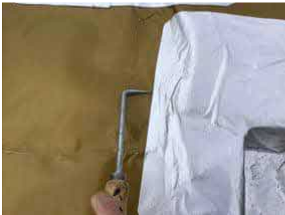
Plot 5 pick testing all SAGM detailing.
