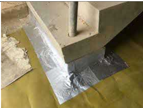
Retro fit detail using SAGM to the base of the concrete stairs in apartment block b.
