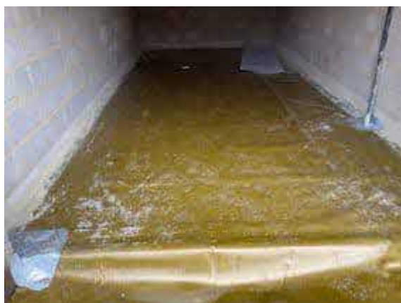
Overview of Visqueen HC Blok infill installation to Plot 32 FOG Unit Garage.
