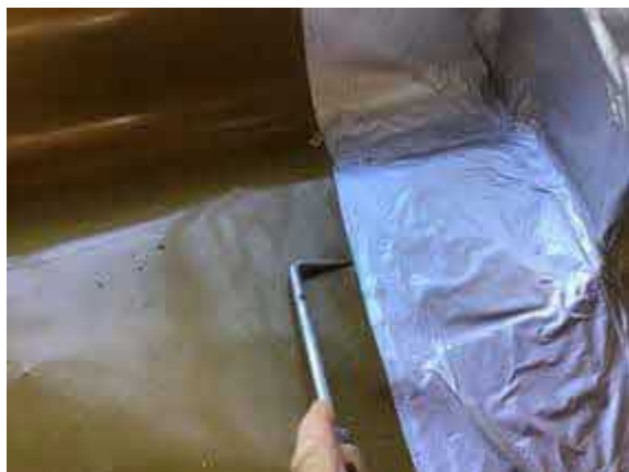
Plot 3 pick testing all SAGM detailing.
