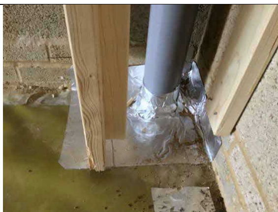
Sealed pipe penetration using SAGM to the rear of the garage plot 45.
