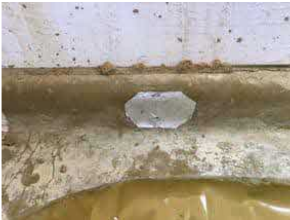
Plot 32 patch repair to damaged membrane caused by follow on trades and repaired using SAGM.
