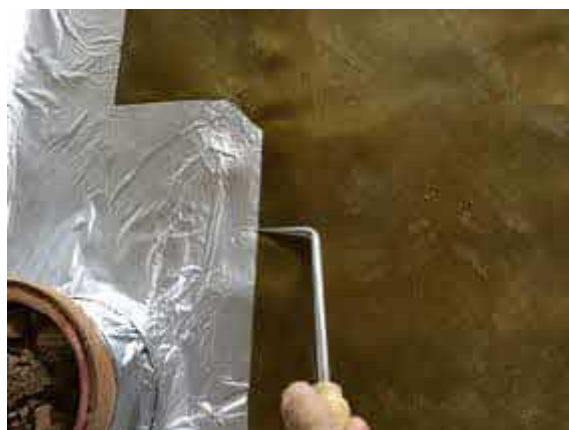
Plot 28 pick testing all SAGM detailing.
