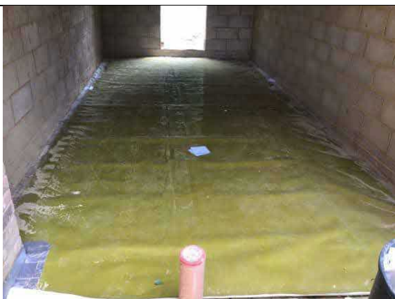
Overview of installed membrane to the garage, as an infill to plot 69.
