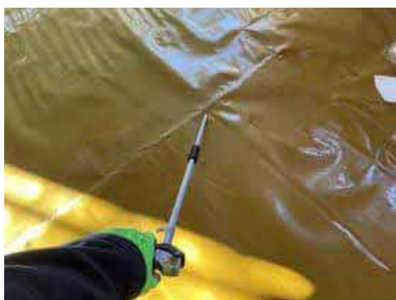
Plot 73. Air lance integrity test conducted upon all hand welded membrane lap joints.
