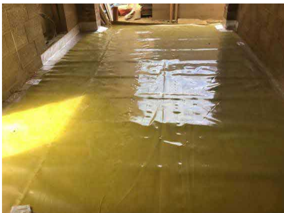
Overview of installed membrane to the garage, as an infill to plot 71.
