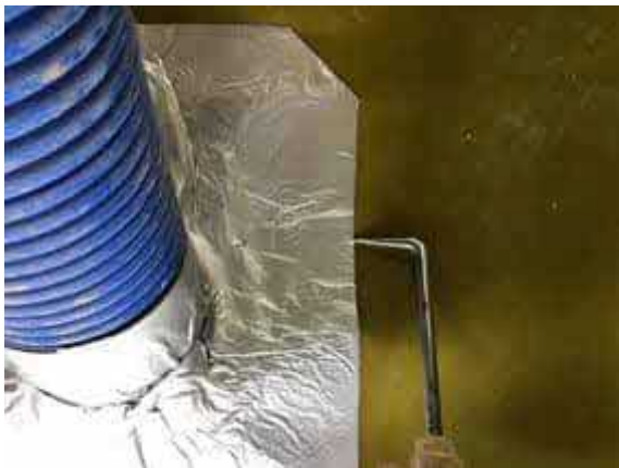
Pick testing all SAGM detailing in plot 50.
