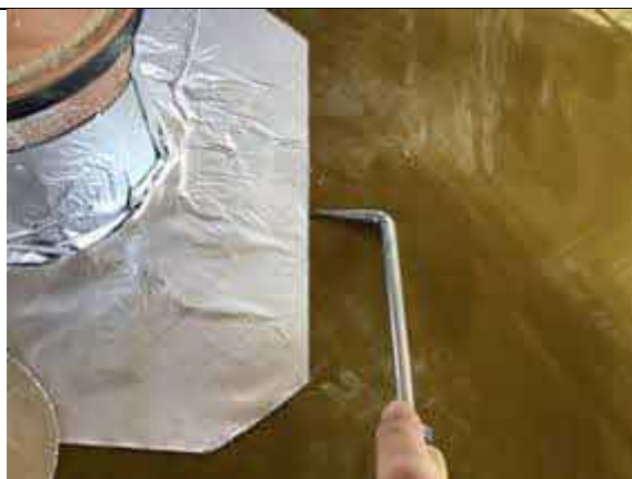
Plot 76 pick testing all SAGM detailing.
