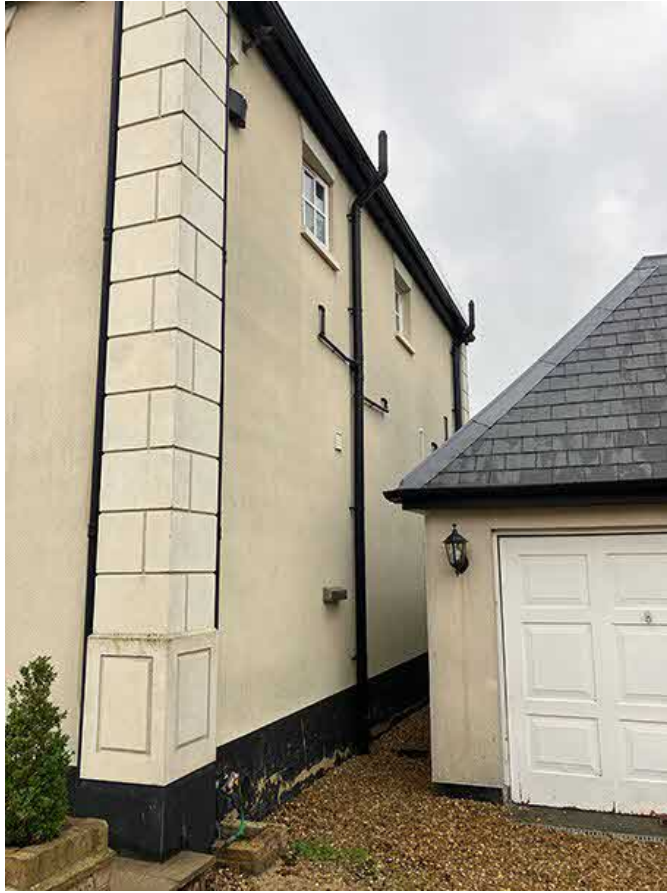
Above: View of corridor between garage and the main house where the minimal glass link is proposed
