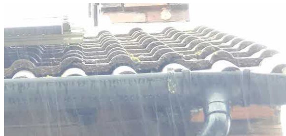
4 Example gaps under tiles on south aspect
