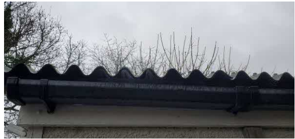
12 Gaps under roof corrugations
