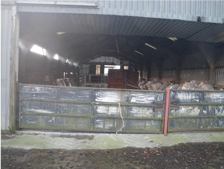
Sheep Shed 1 is empty apart from the temporary storage of recycled materials.
