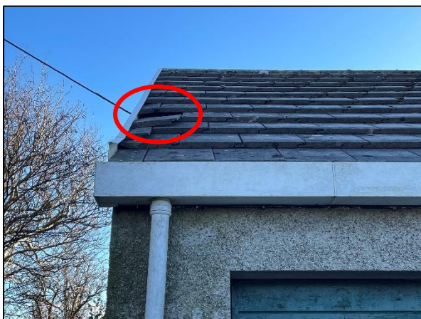
Figure 5 Damaged tile on garage
