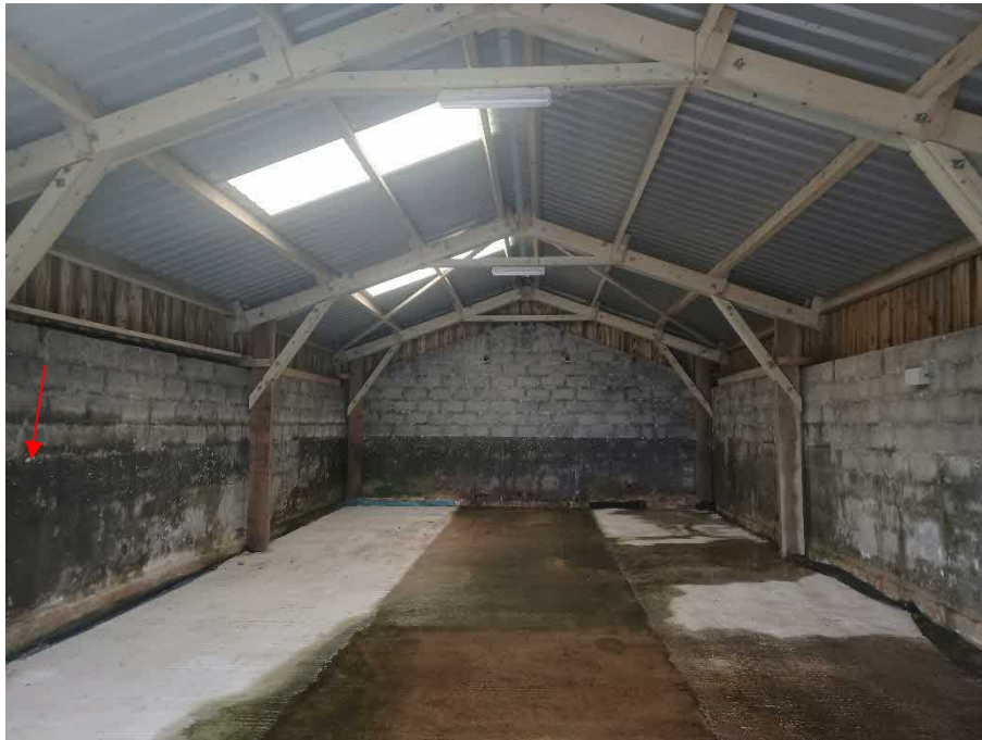
Figure 4: View of interior of Barn 1. Red arrow shows gaps between the block wall top and the wood panels providing potential bat access to the barn interior.
