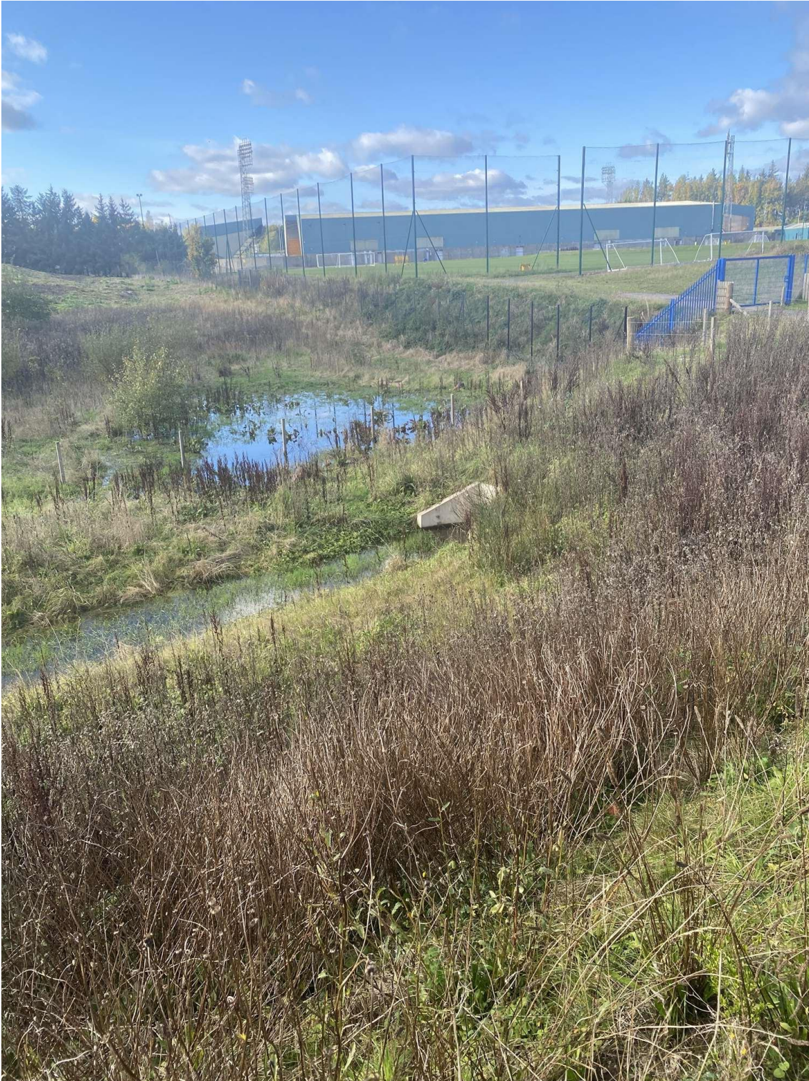
Photo 3: North end of swale showing culvert under access to sports centre and ponding of surface water to west of swale
