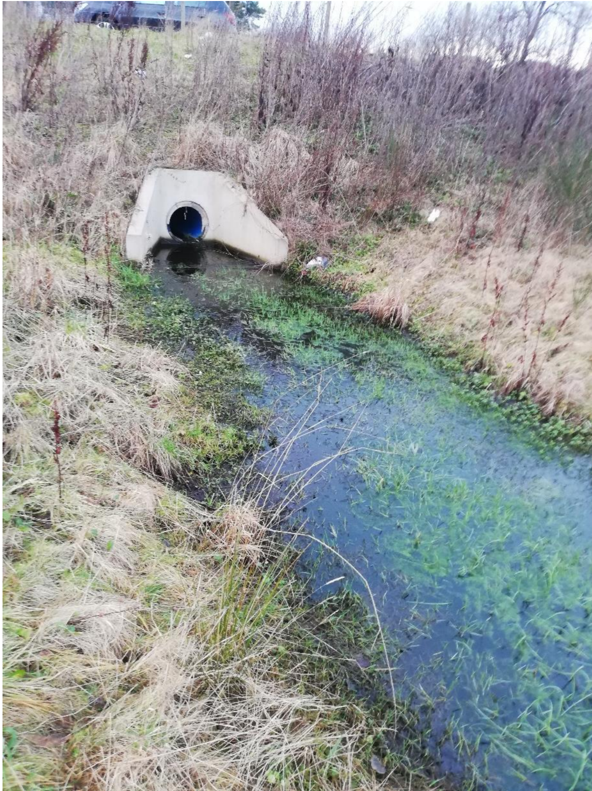
Photo 9: TN5 Culvert with standing boggy water.
