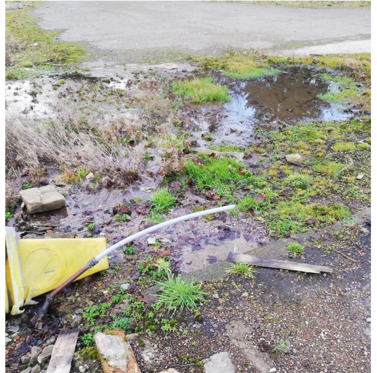
Photo 8: Target Note 1, running water mains tap causing standing water in the hard ground habitat.
