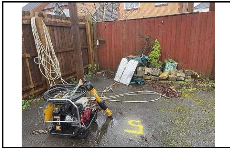
Photo OE/1702/1057/R3/P22 – Location and commencing surface at Window Sample WS5 – at the northeast corner of the site.
