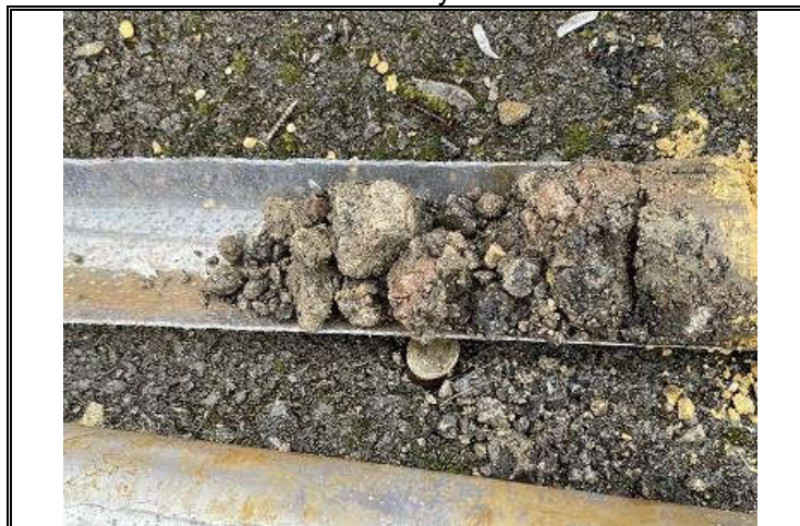
Photo OE/1702/1057/R3/P24 – Window Sample WS5 – Drilling cores 0.07 to 0.2m bgl – Made Ground – rock fill beneath tarmac surfacing.
