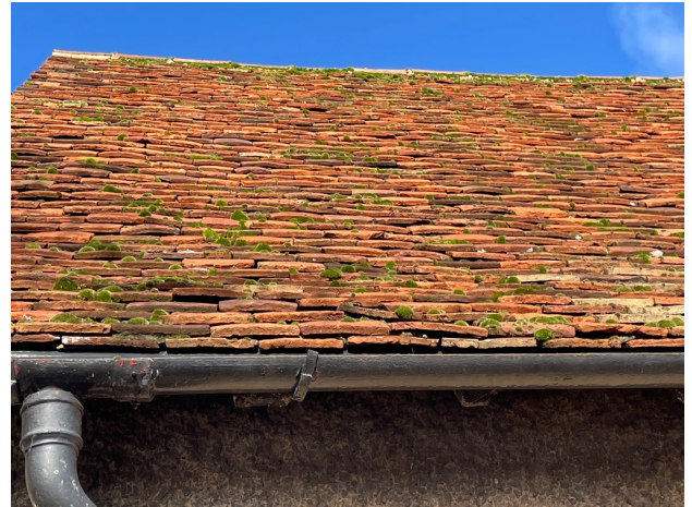
Photograph 4: Gaps under roof tiles.
