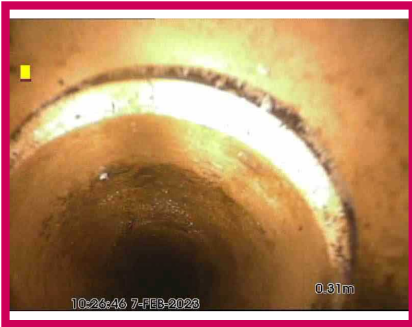
1, 00:00:13, 0.40 m Joint displaced, medium
