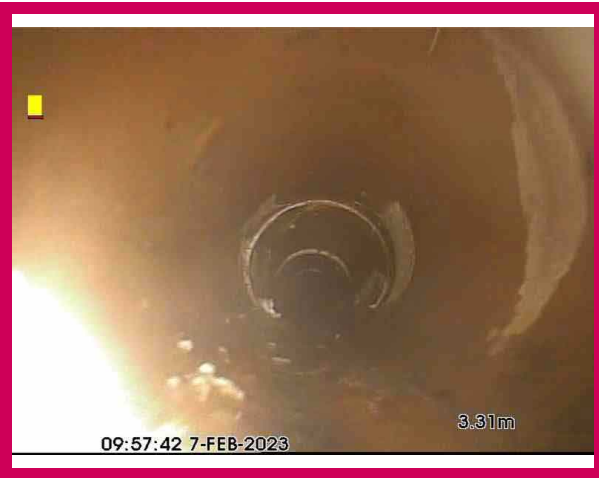
1, 00:00:15, 3.31 m Crack, circumferential at joint from 12 o'clock to 12 o'clock
