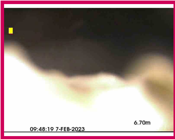
1, 00:00:23, 6.70 m Attached deposits, fouling from 3 o'clock to 9 o'clock, 30% cross-sectional area loss
