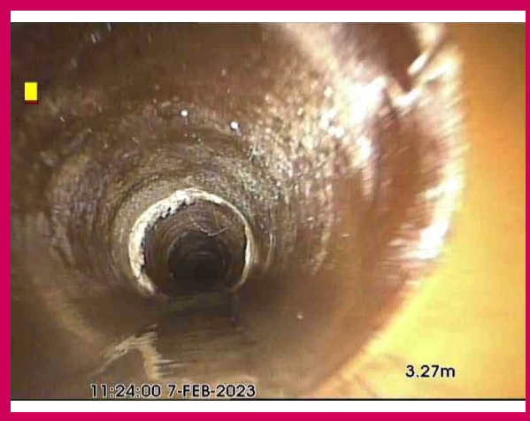
1, 00:00:15, 3.37 m Crack, circumferential at joint from 12 o'clock to 12 o'clock
