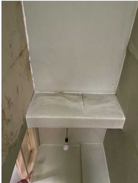
Photograph 12. Timber Lintel Supporting Wall Above Top of Stairs
