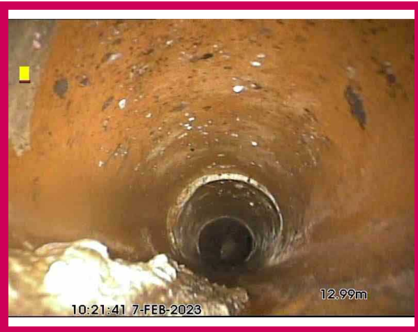
1, 00:00:37, 13.00 m Attached deposits, fouling from 3 o'clock to 9 o'clock, 10% cross-sectional area loss
