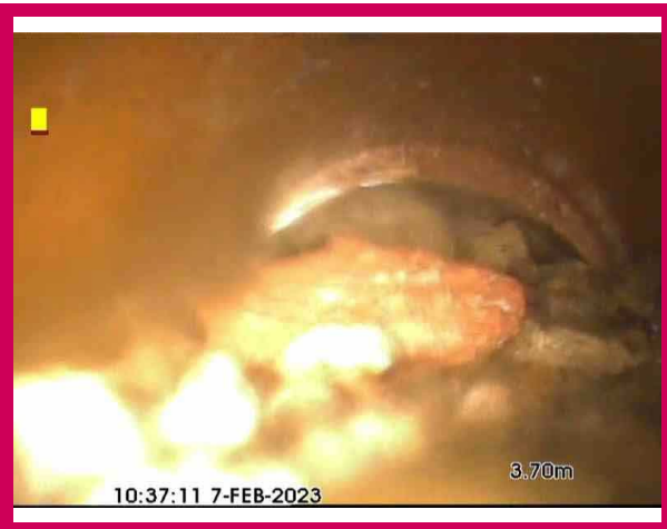
3, 00:00:21, 3.91 m Settled deposits, hard or compacted, 100% cross-sectional area loss
