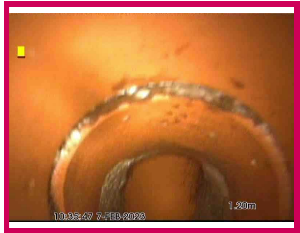
2, 00:00:11, 1.24 m Crack, circumferential at joint from 12 o'clock to 12 o'clock
