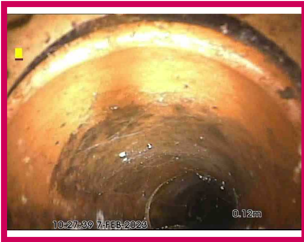
1, 00:00:05, 0.14 m Joint displaced, medium
