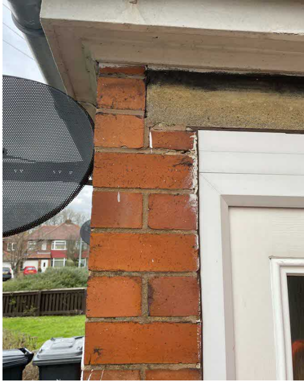
Photograph 15. External Wall to Porch Leaning Out
