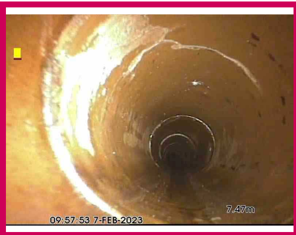
3, 00:00:27, 7.45 m Crack, circumferential at joint from 12 o'clock to 12 o'clock
