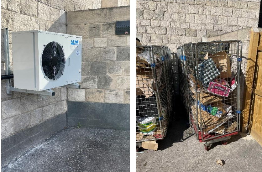
The position of the condenser (left) and the area's previous use as storage for refuse cages (right).
