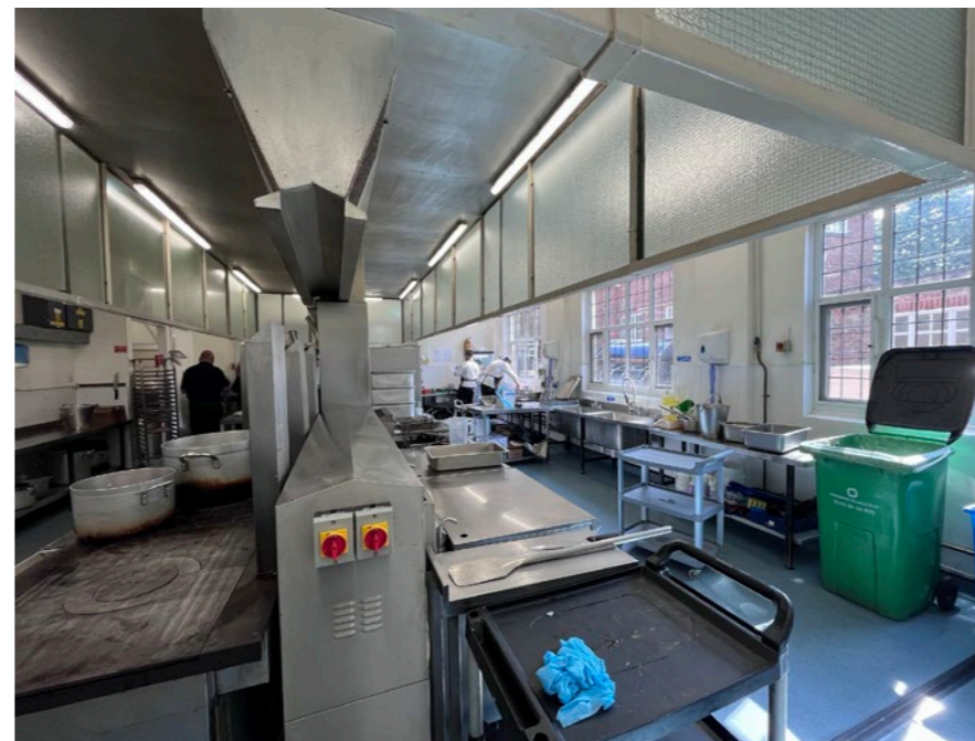
existing kitchen equipment at the end of useable life
