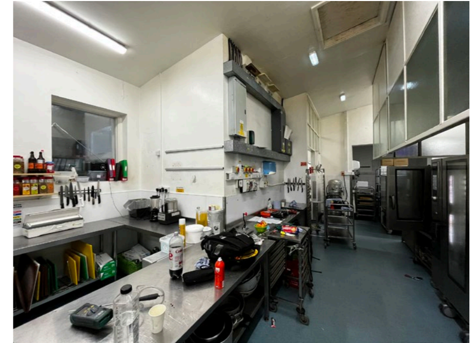
existing kitchen equipment at the end of useable life
