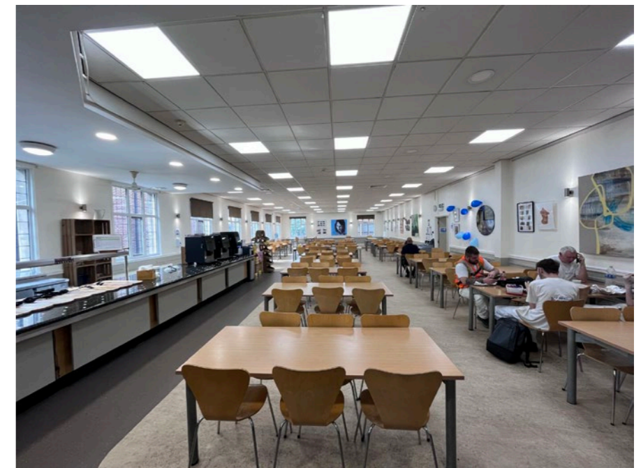
existing level surface across the dining hall, step at far end to be removed
