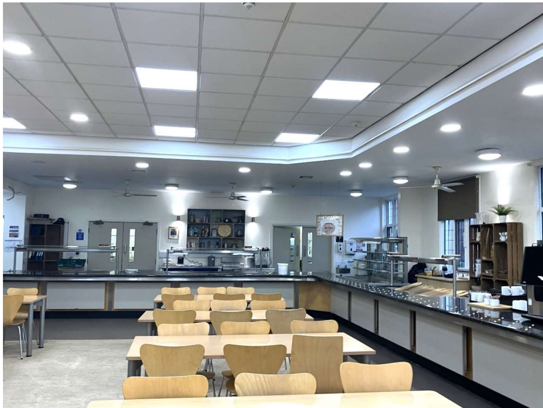
VIEW FROM DINING AREA TOWARDS EXISTING SERVERY SHOWING WALL AND DOORS BEHIND SERVERY TO BE REMOVED & SUSPENDED CEILING RE-CONFIGURED; WALLS & FLOOR MADE GOOD/RECOVERED
