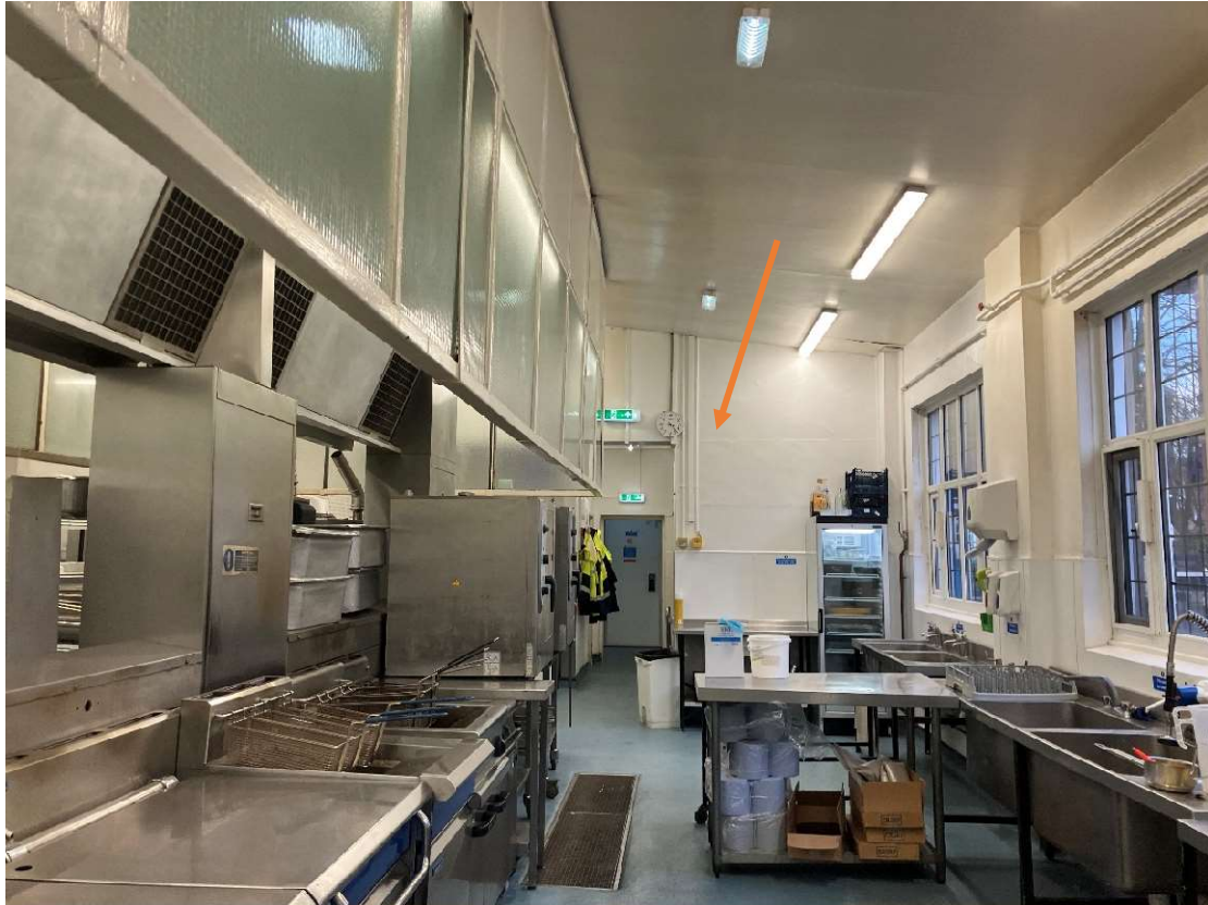
VIEW LOOKING SOUTH WITHIN KITCHEN TO PARTITION WALL TO BE REMOVED. NOTE WINDOW ON RIGHT WILL BECOME PART OF THE EXTENDED DINING AREA
