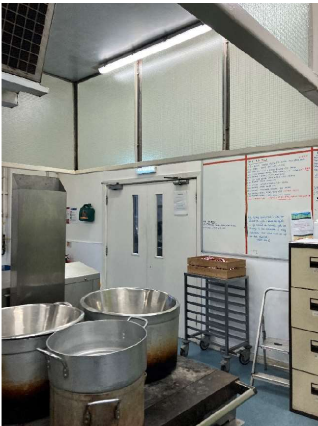
DETAIL OF DOORS AND PARTITION TO BE REMOVED, VIEWED FROM KITCHEN SIDE
