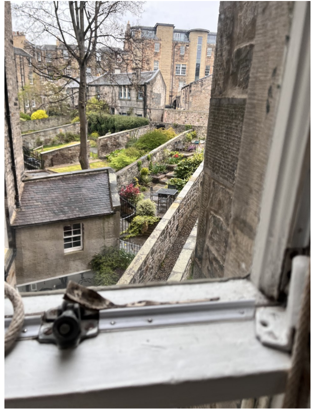
Window sash out of alignment causing weak contact points at mid transom, top sash and bottom sash, allowing major draughts to enter the property. Has been retrofitted with inadequate face fixed brushes.
