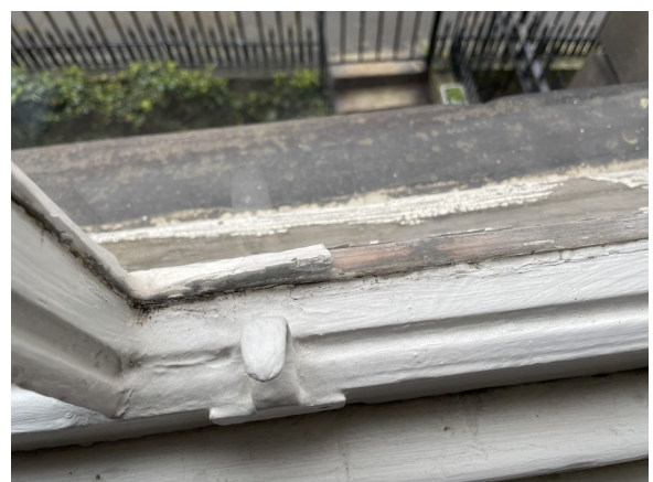
Defective sections of timbers require to be replaced.
