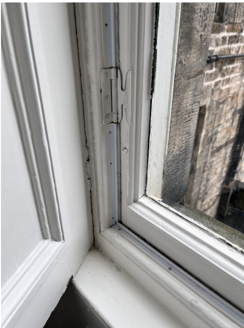
Defective easy clean battens and ironmongery requires replacement.
