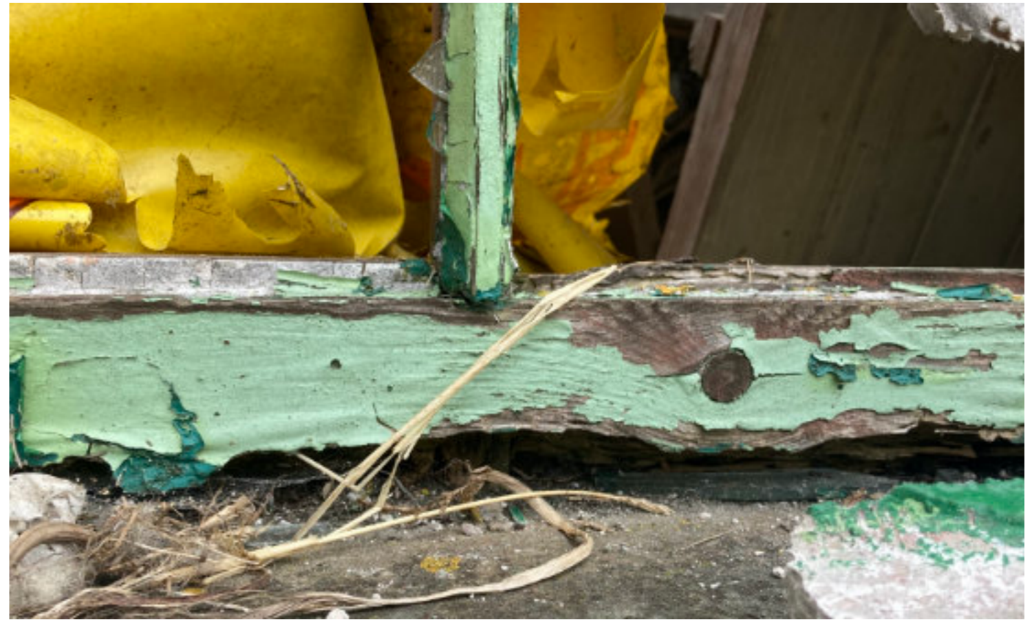
Timber framing to windows have widespread rot damage
