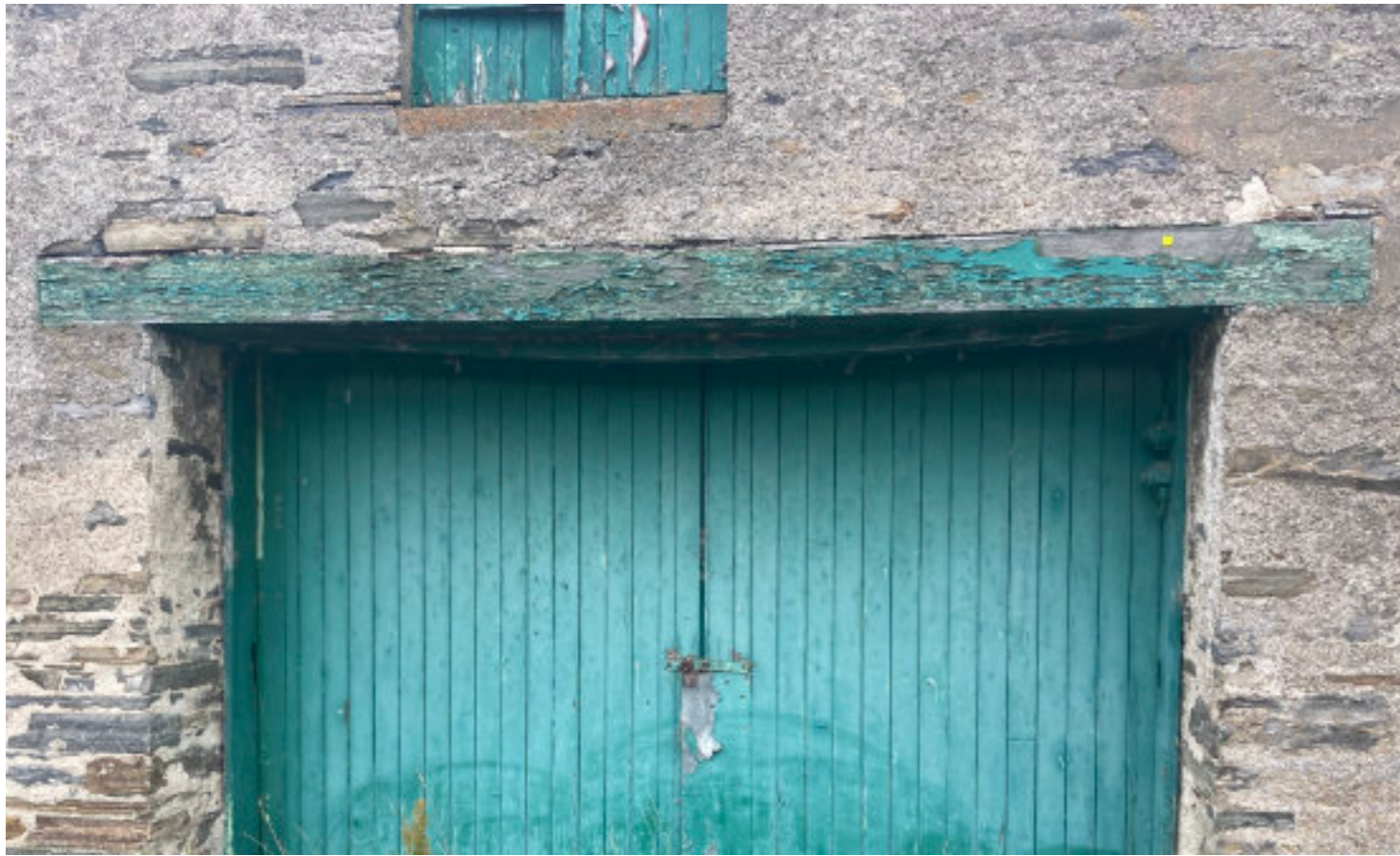
Timber lintol to East elevation showing signs of failure. Internal lintols have completely failed.
