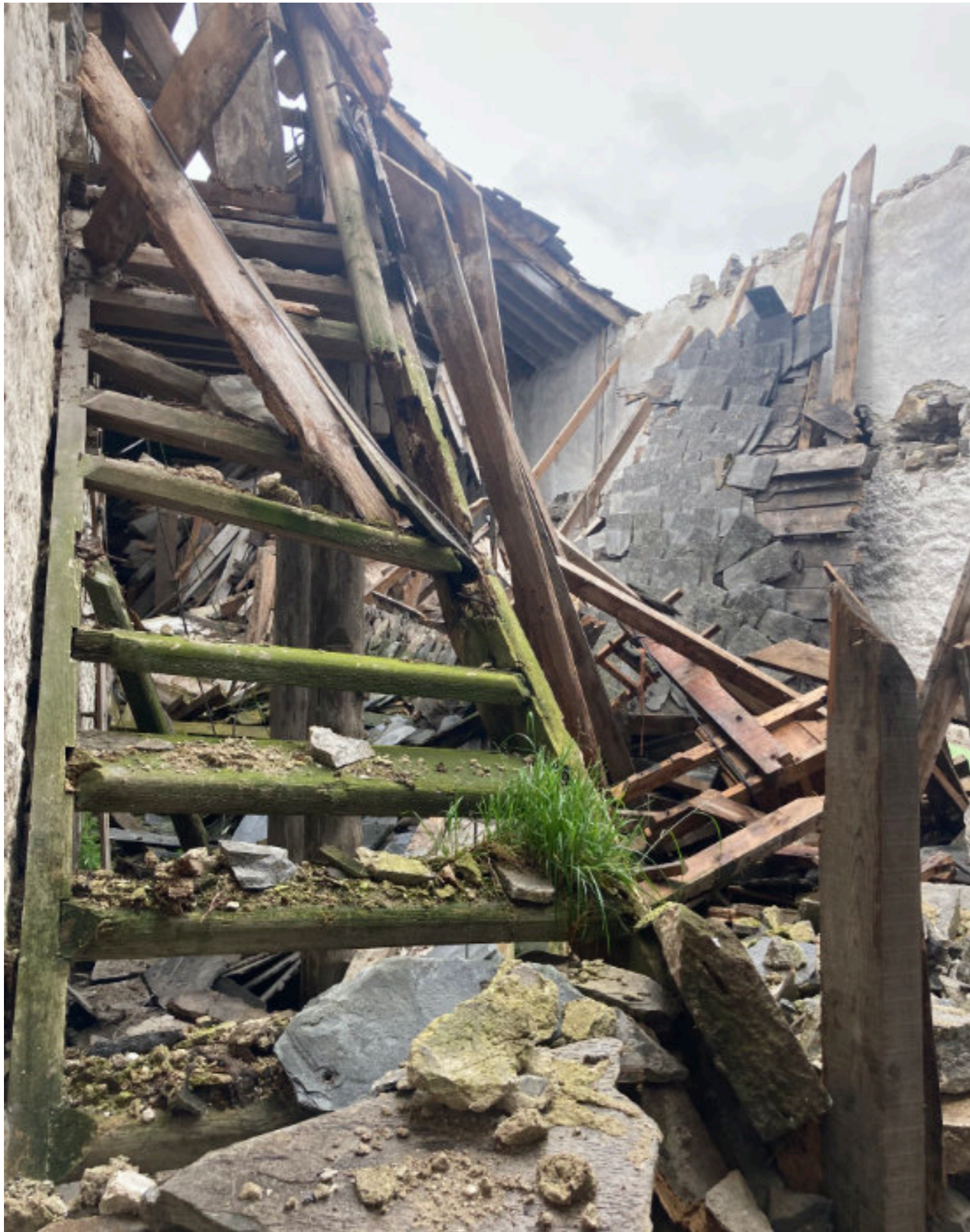
Interior of area where roof has collapsed - note all timbers beyond retention
