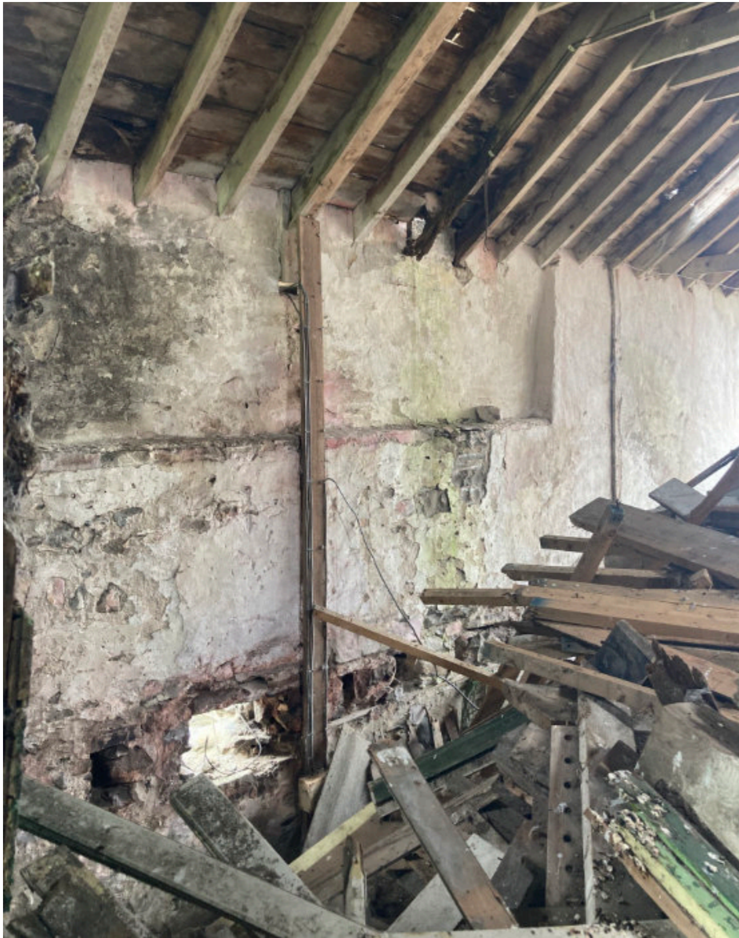
Evidence of external wall adjustment - this relates to exposed gable on North elevation
