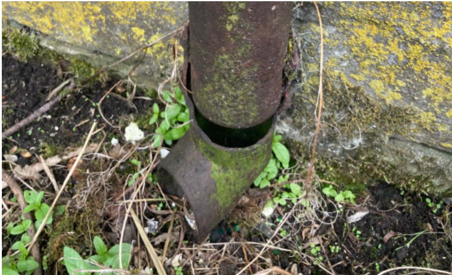
Existing cast iron rainwater goods appear to have corroded beyond repair
