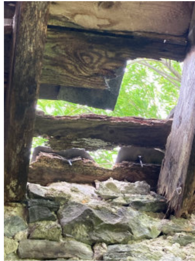
Condition of sarking/existing timbers to remaining roof.
