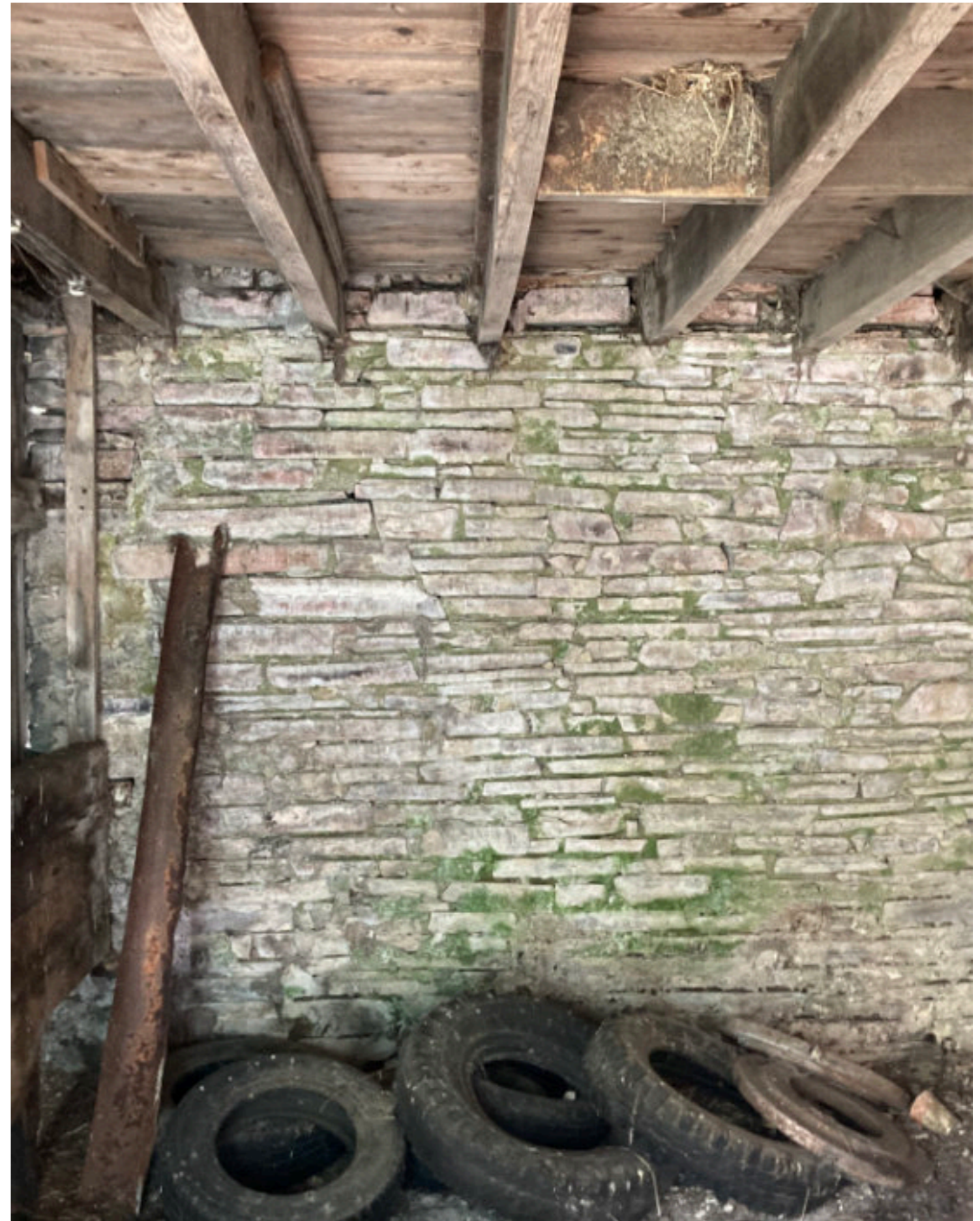
Ground floor accessed at South elevation. Note stone appears to have been exposed
