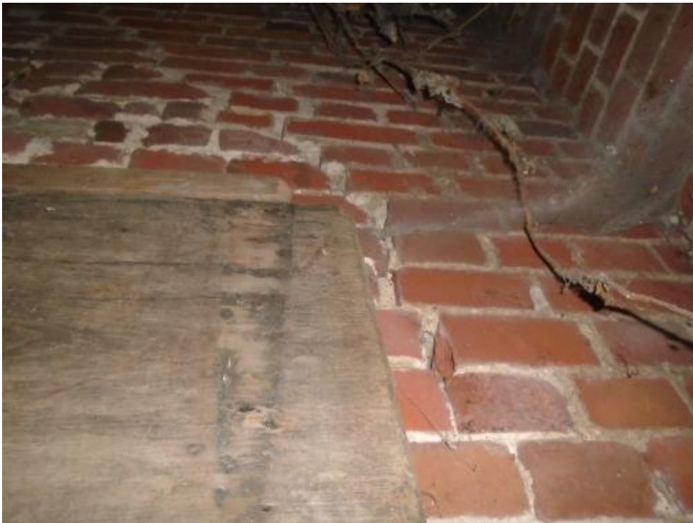
Photo 8. Example of cracks within the brickwork.
