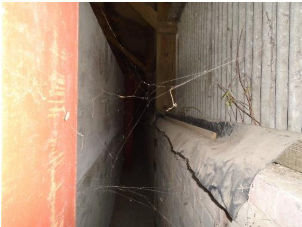
Photo 4. Void between the internal and external wall.
