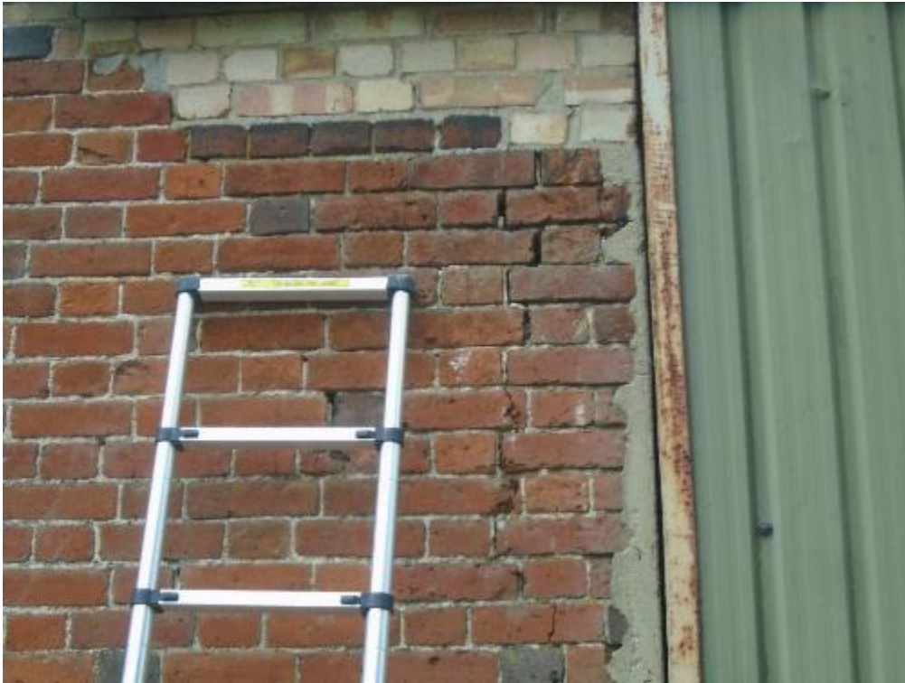
Photo 9. Example of cracks within exterior brickwork and gaps between the door frame.
