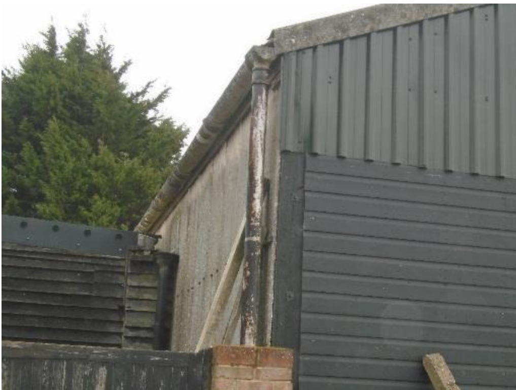
Photo 2. Cement fiber sheeting and wooden cladding on north and west elevations of barn.
