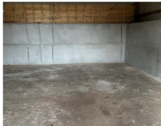
Image 12: Exposed concrete slab internally @ northwest corner
