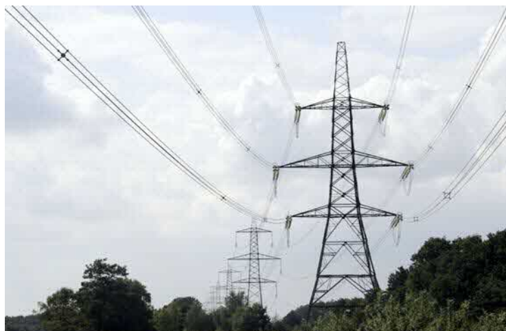
Figure 1 275 kV transmission line
