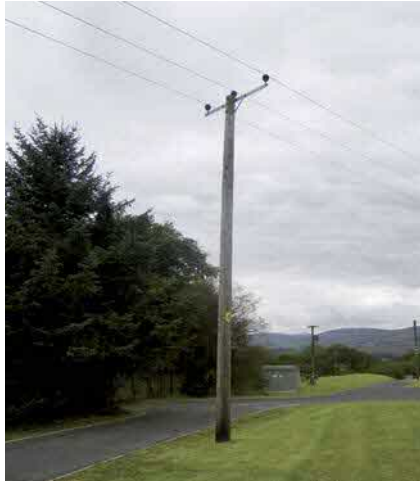
Figure 2 11 kV distribution line
