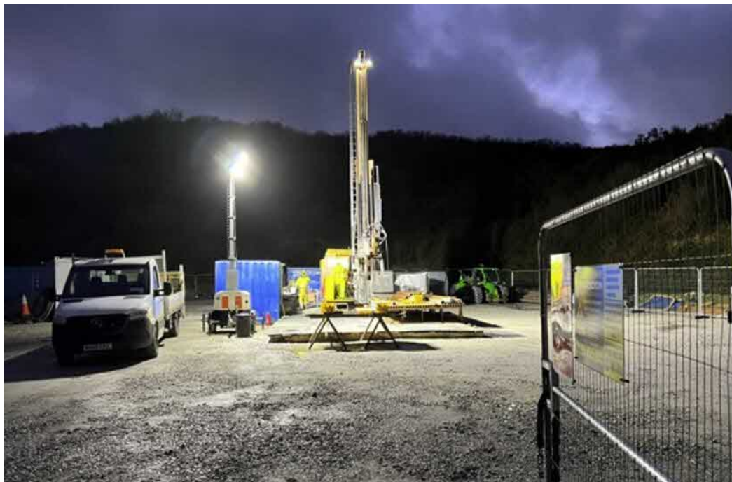
Appendix 2: Example of the DBC S25 drill rig which Cornish Lithium plan to use for this mineral exploration drilling programme. A drill rig with similar specifications may be used.
