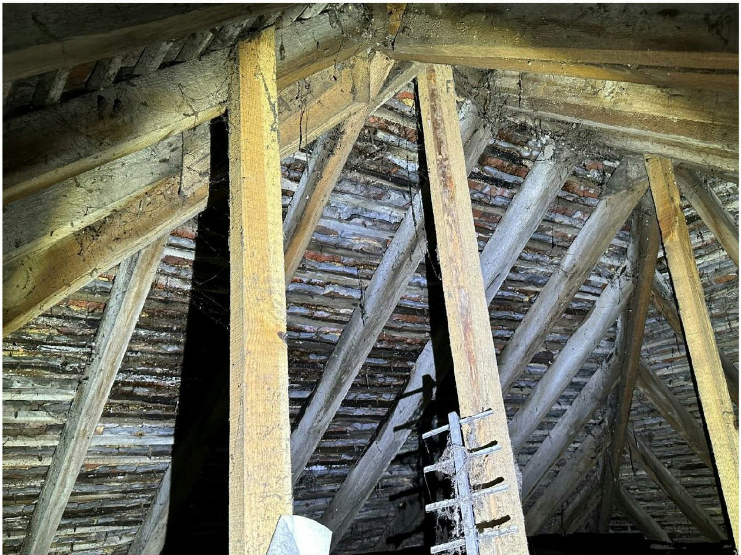
Photos showing existing roof problems
