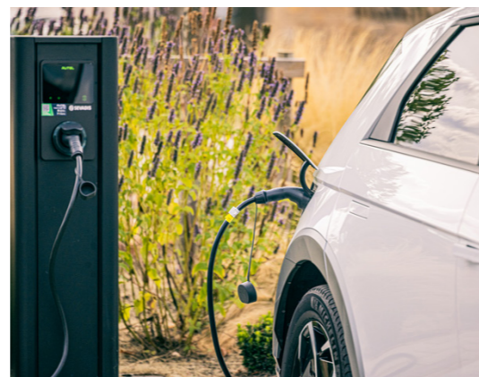
Figure 38. Electric Vehicle Charging
