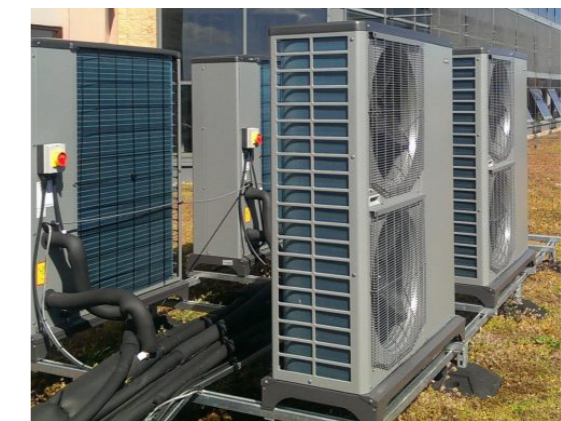
Figure 40. Rooftop air source heat pump
