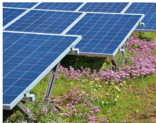
Figure 37. PV Panels over biodiverse roof
