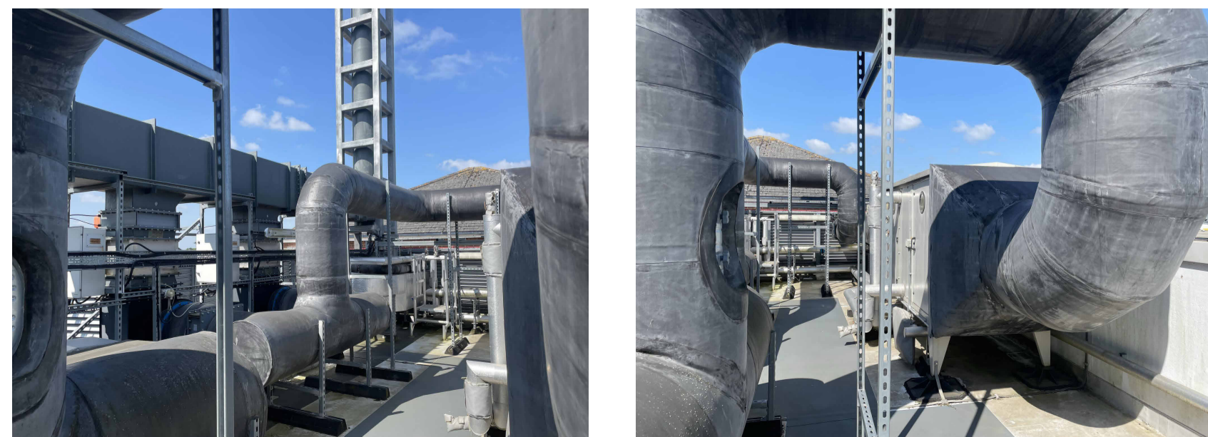
IMAGE 03 & 04 - EXISTING AIR HANDLING UNIT AND DUCTWORK
