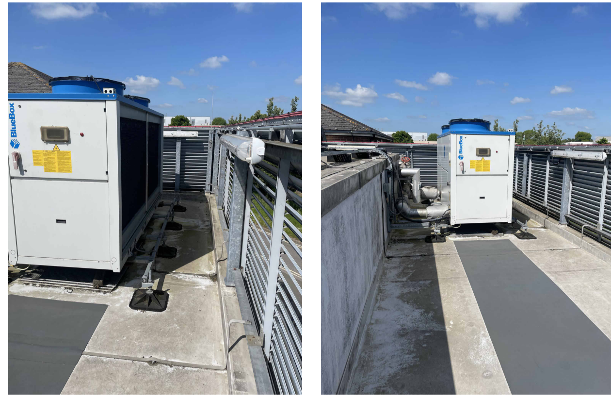
IMAGE 01 & 02 - EXISTING CHILLER UNIT AND VACANT AREA FOR PROPOSED CHILLER
