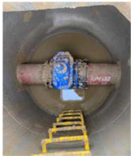
Shut-off Valve Chamber
