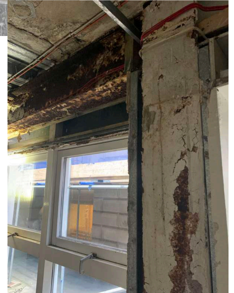
The tanking at street level does not cover the full extent of the basement so water has been entering the building via the concrete slab and reaching the steel structure which is in poor condition with extensive areas of rust.
