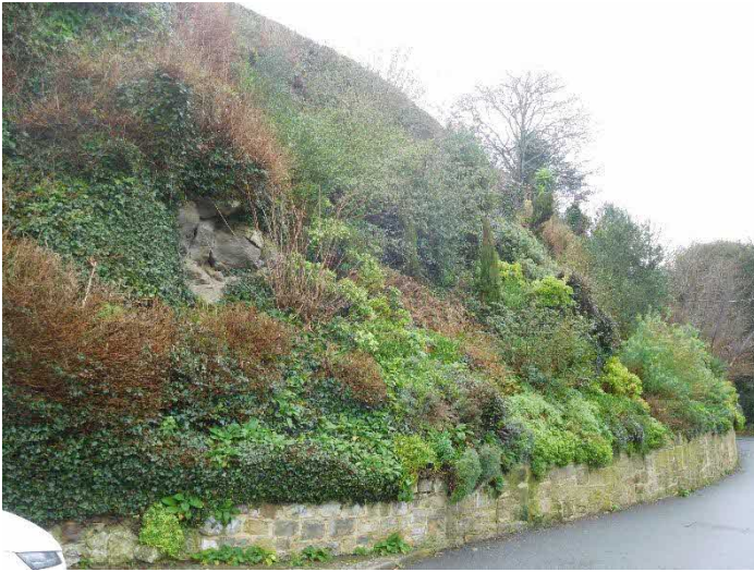
View of slope and low stone wall along southern boundary of the site with Undercliff Gardens - Note: rock outcrop
