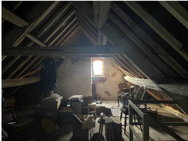
Plate 4 – Farmhouse, internal roof void
