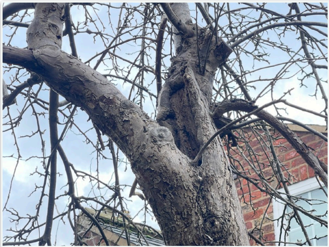
Figure 2. Open cavity at the main bifurcation which extends down to ground level.
