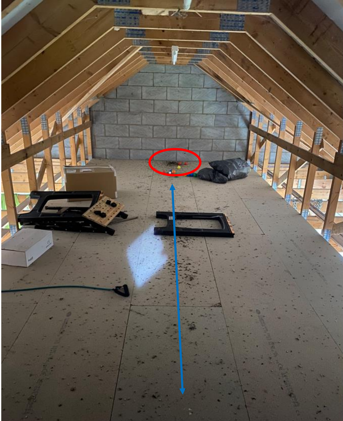
Plate 3: Partially boarded roof void with red circle showing BLE droppings on western gable and blue line showing LHS droppings beneath ridge.
