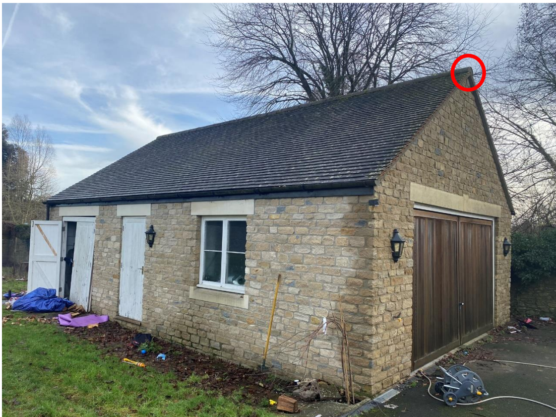
Plate 2: Side (N) and front (W) elevation of the garage. Red circles indicates likely roosting area for brown long eared bats.
