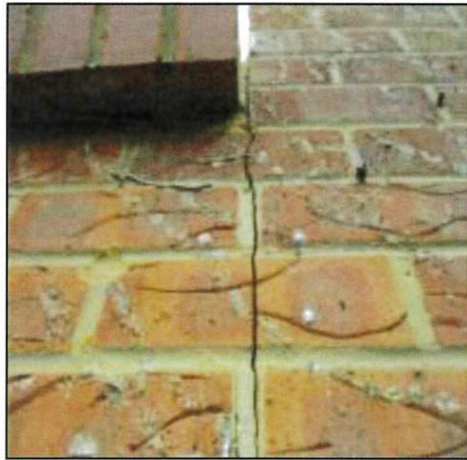
Figure 4. Photograph of vertical crack below first floor window.
