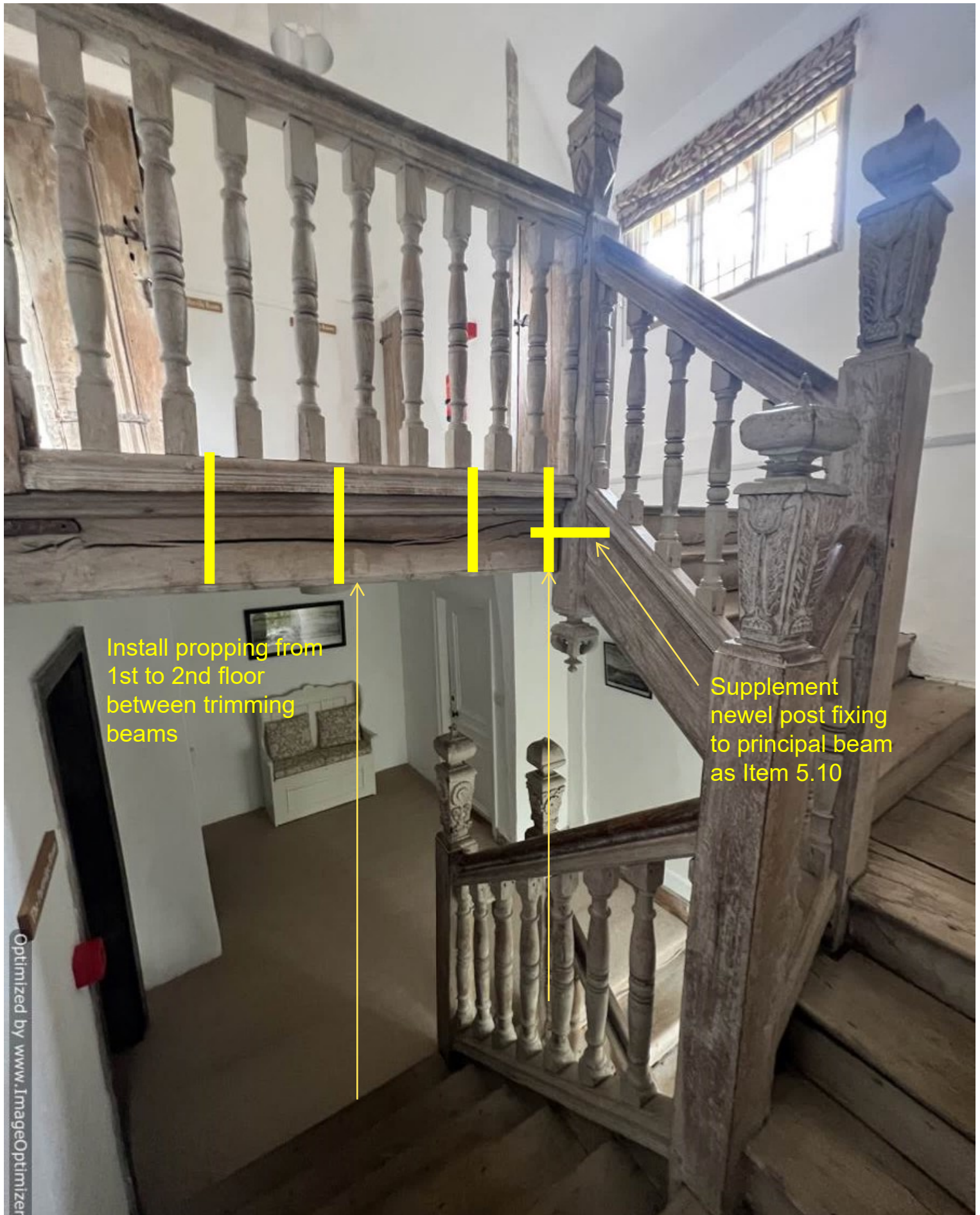
Photo 4 - 2nd floor stairwell. Principal trimming beam to repaired.
