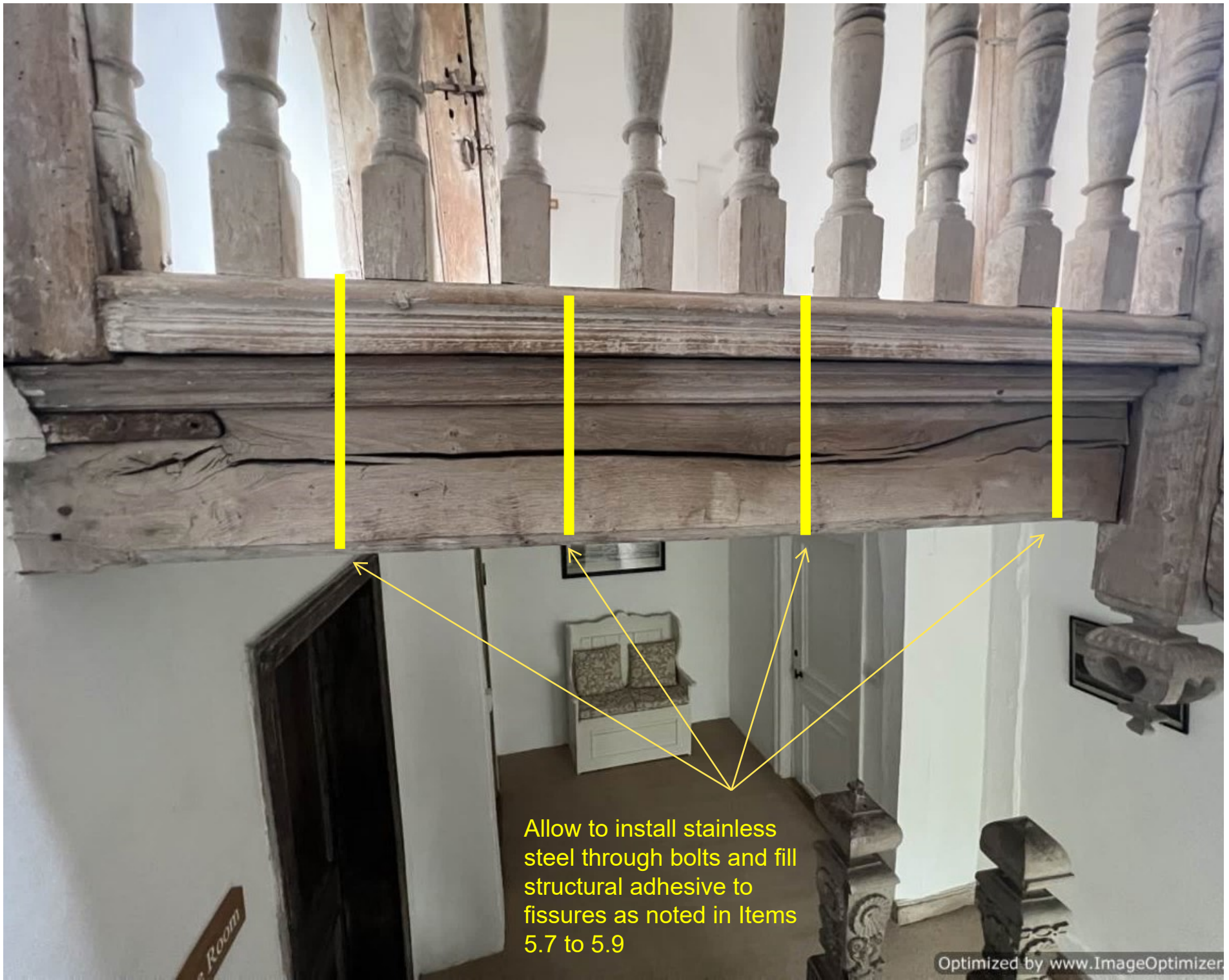
Photo 5 - 2nd floor stairwell trimming beam to be repaired.
