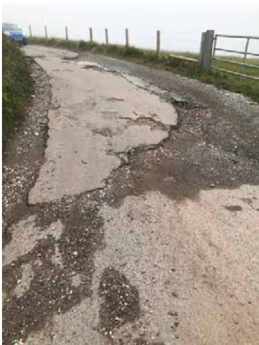
Figure 12 Condition of the Access Road in 2021, prior to repair
