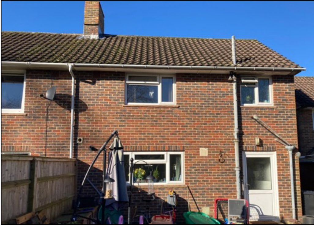
Photograph 1. The rear elevation of the property. Note the intact tiles, brickwork and sealed soffit boxes.
