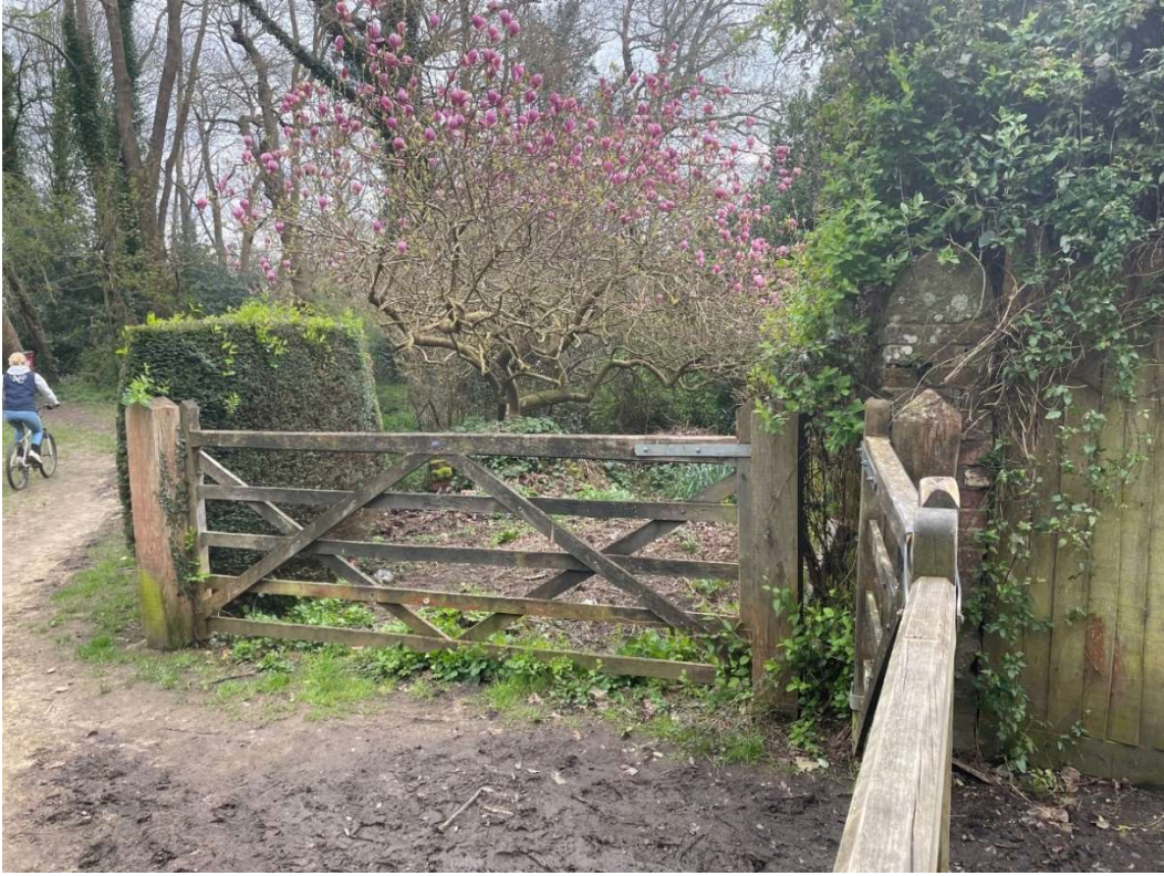
Vehicular cross over: The existing vehicular and pedestrian crossover is in very poor condition. The suggested proposal is the extend the existing road Tarmac into the crossover.
