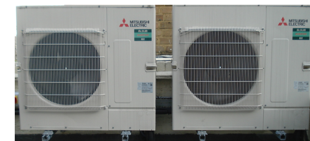
Proposed External Condensing Units
