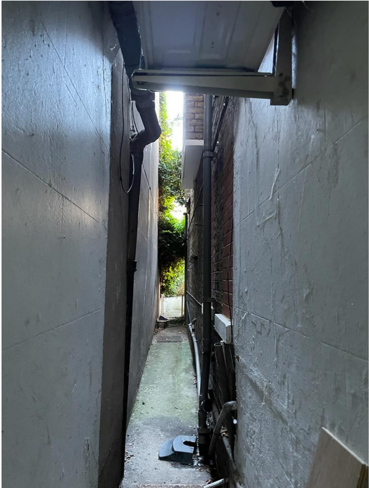
Photograph 6 – Narrow concrete alleyway with two rectangular manhole covers, located along the eastern boundary.
