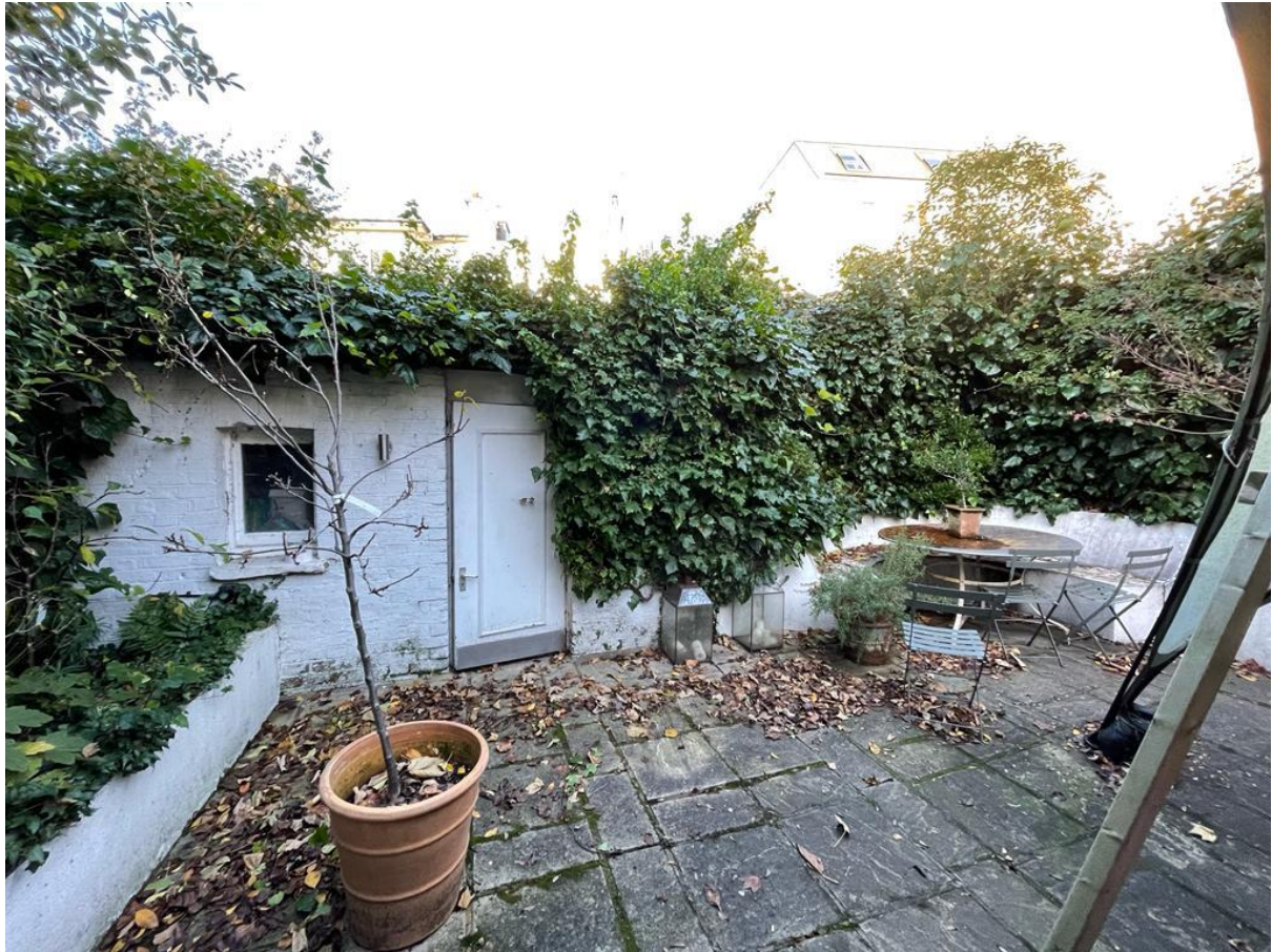
Photograph 9 – Single-storey brick structure located in the far north of the rear garden.
