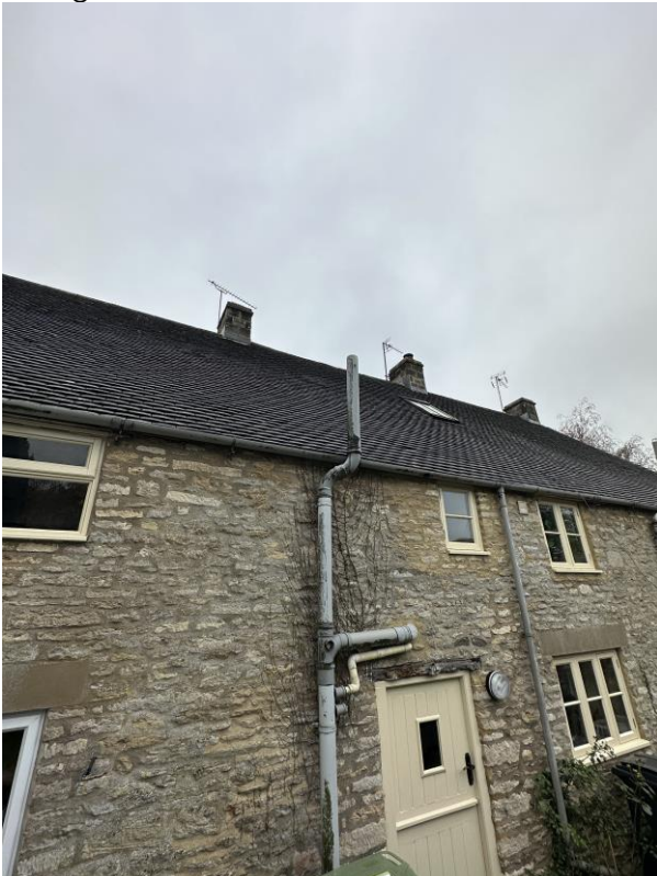
Photograph 4 – View showing rear elevation No. 11 with purpose made windows and conservation rooflight.
