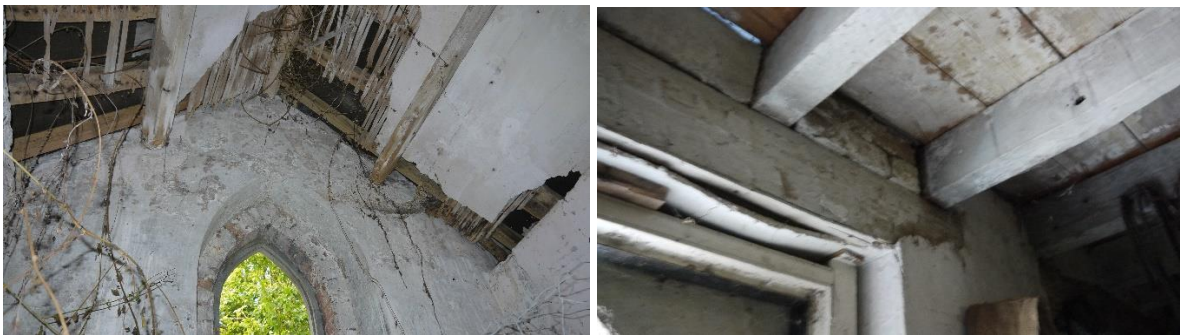
Plate 8 (left) first floor ceiling and lath and plaster failing and plate 9 (right) first floor timber floor joists.
