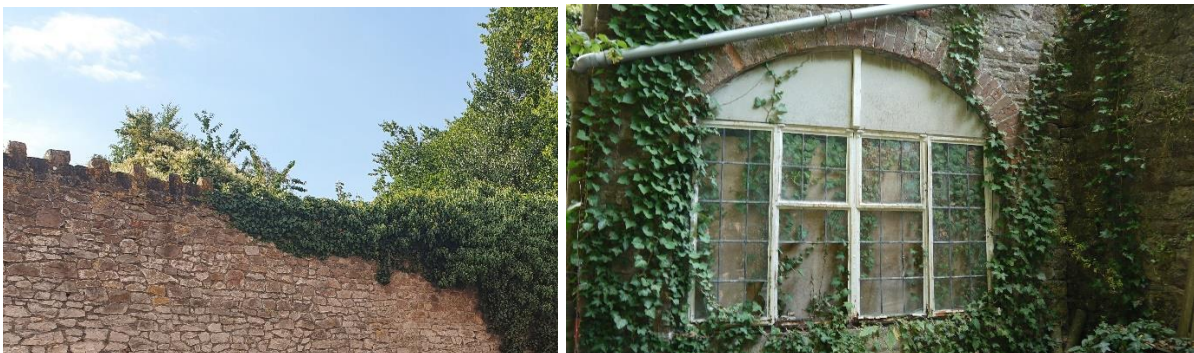
Plate 6 (left) Boundary wall crenellations to the site and plate 7 (right) blocked in window.
