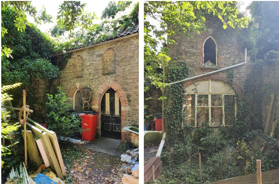
Plate 2 (left) The Folly front elevation. Plate 3 (right) Side façade of The Folly.
