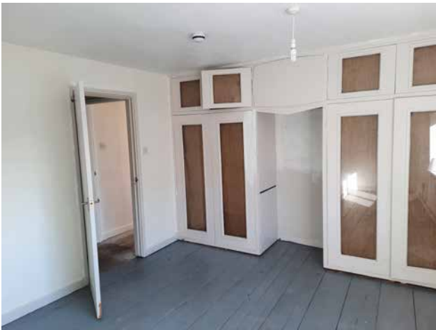
3.45a First floor rooms with no historic features other than original floorboards
