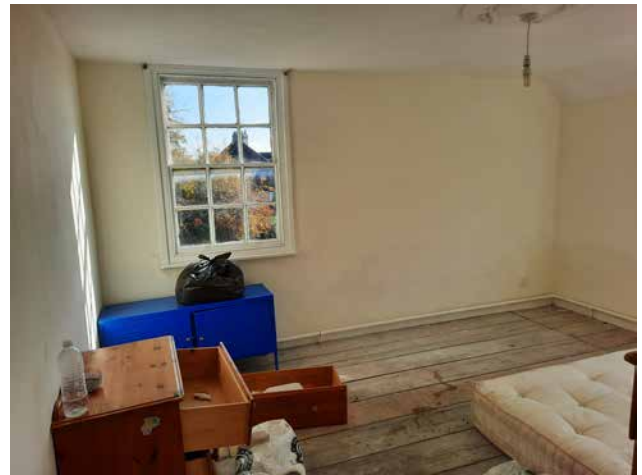
3.45b First floor rooms with no historic decorative features, modern stud partition
