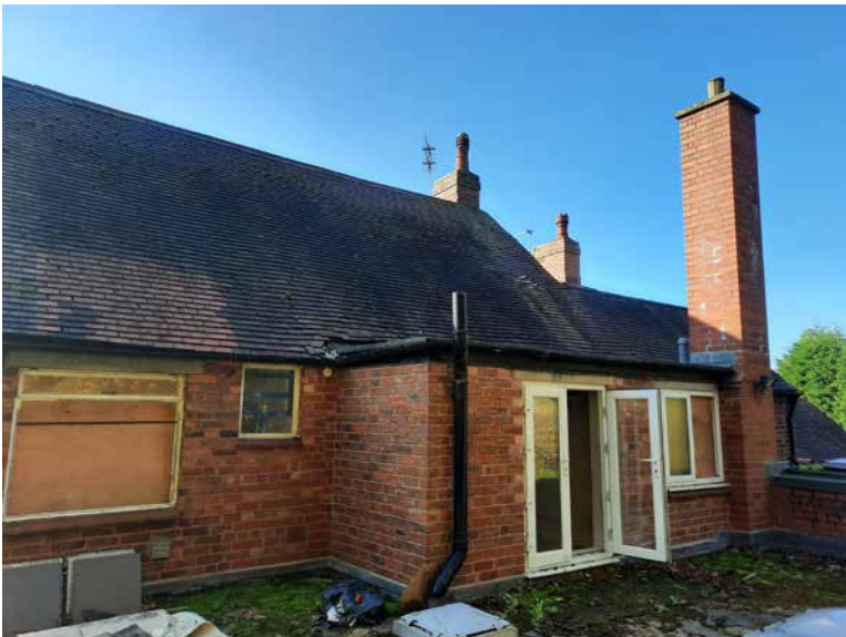
3.34b First floor rear facade-staircase enclosure with modern door, windows and lintels
