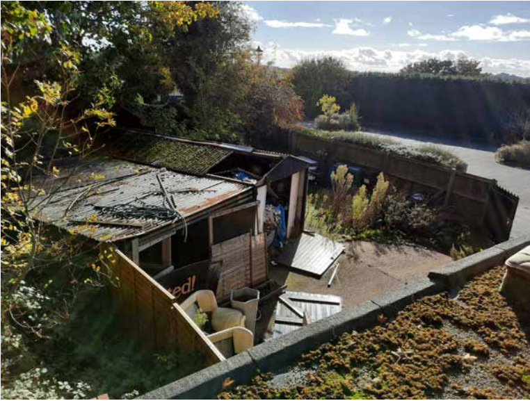
3.25 Dilapidated outbuildings and hard landscaping to the east side
