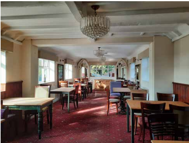
3.38 Single storey wing projecting to east, original wall and timber beams evident in first bay
