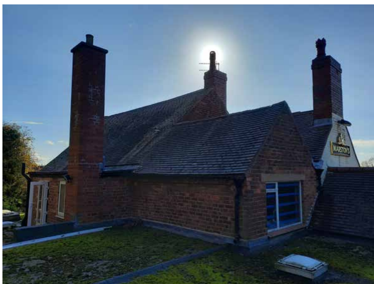
3.30 Roof line of pitched roof, lower M pitched roof and projecting pitched roof single storey wing
