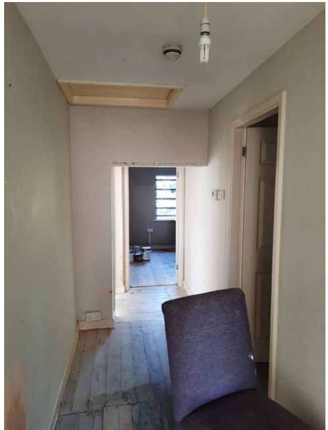
3.44b Central corridor at first floor with modern stud partitions and opening through original external wall
