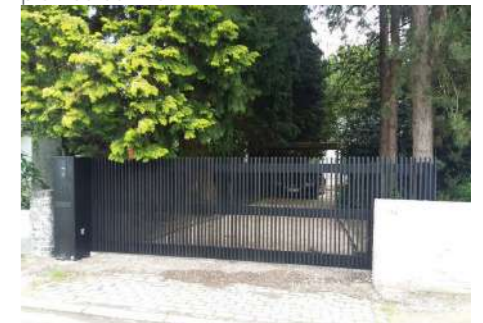
3.7.3 Electric metal sliding gate
