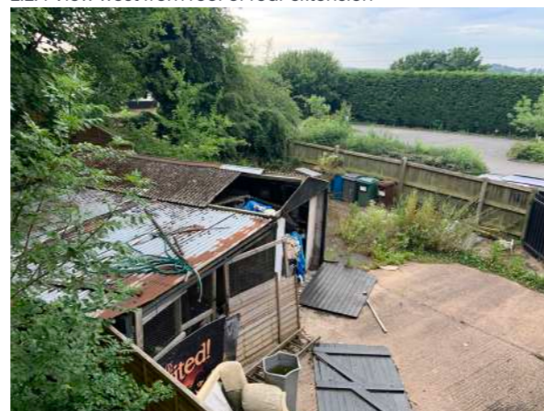
2.2.7 View from roof into service yard to east with car park to south
