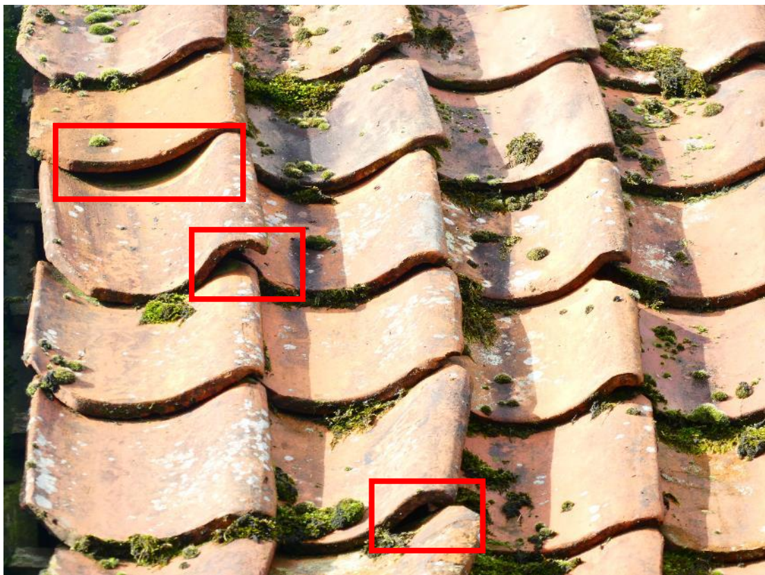
Photo 5, gaps under lifted roof tiles (highlighted in red) on building one.
