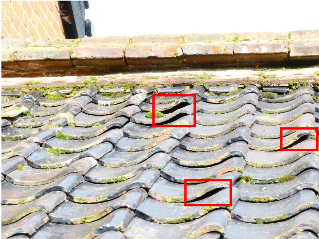
Photo 9 , gaps under lifted tiles (highlighted in red) on section A.
