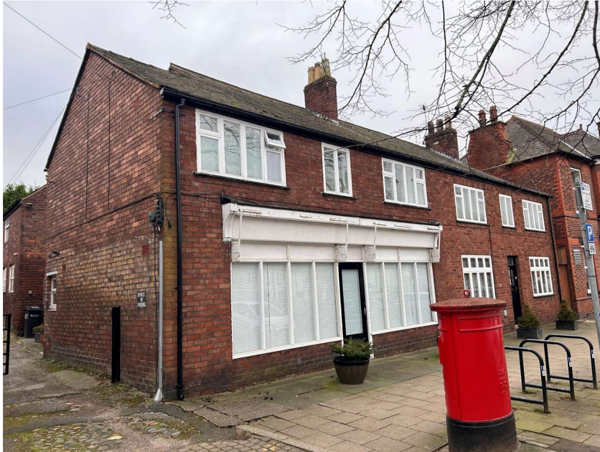
Existing front elevation, showing existing shop front and attached neighbouring residential property front facade
