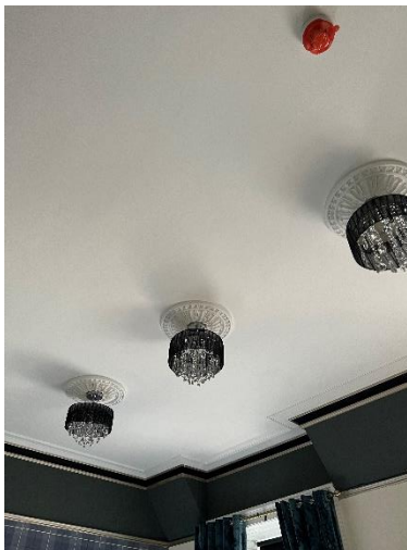
Suite 02 2 nd floor ceiling roses and smoke detection
