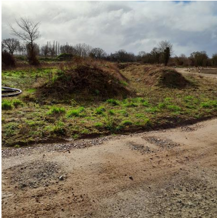
Photo 17. Soil bunds east of access road near junction with loop hardstanding, February 2023.
