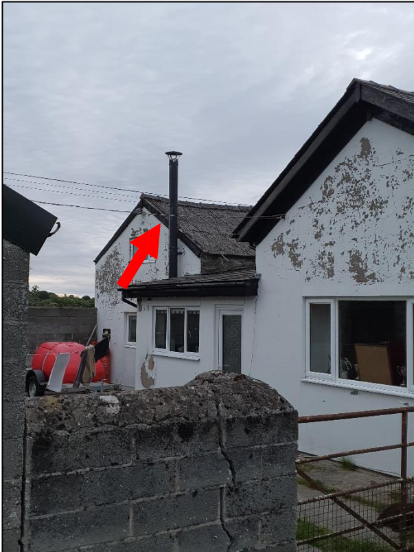
Plate 1: View of the NW elevation of the house from the SW with identified soprano pipistrelle roost indicated behind fascia
