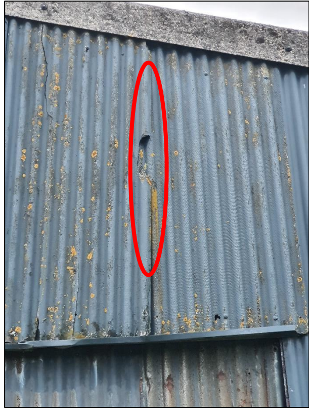
Plate 7: Closer view of the roost location in an overlap of two fibre cement panels
