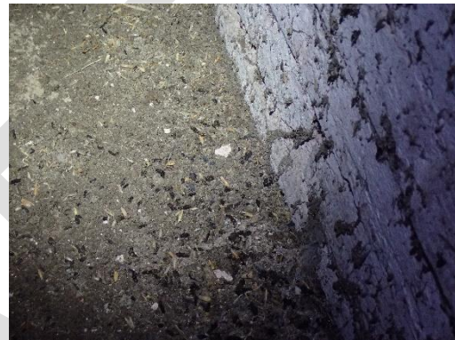
Figure 13. Mixed droppings upon the mezzanine floor within the central section of the barn
