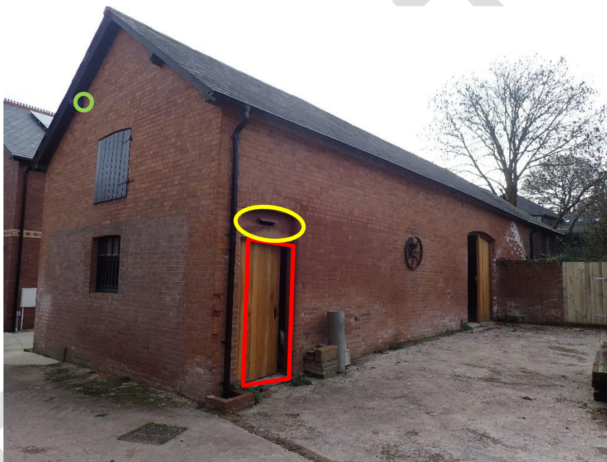
Figure 16. Lesser & greater horseshoe bats observed emerging from doorway (highlighted in red and yellow) and individual long-eared emerging from wall-top (green)
