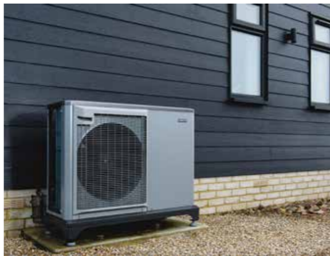
Sustainability Technologies - Air Source Heat Pump
