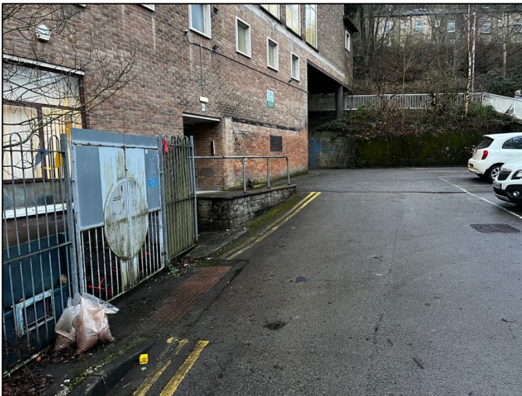
General view to the west along north elevation of the building retaining wall at the west of the site
