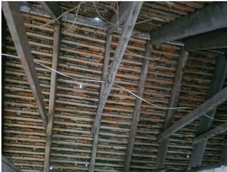
Figure 15: The underside of the roof of B1b, showing bare tiles and tiles gaps where daylight is entering.
