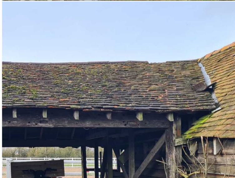
Figure 12: Unsealed and slipped roof/ridge tiles on B1a.
