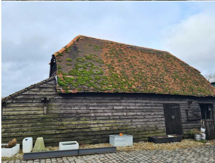
Figure 16: Building B3, showing the eastern elevation. Bat roosting features were incidentally noted across the roof structure.
