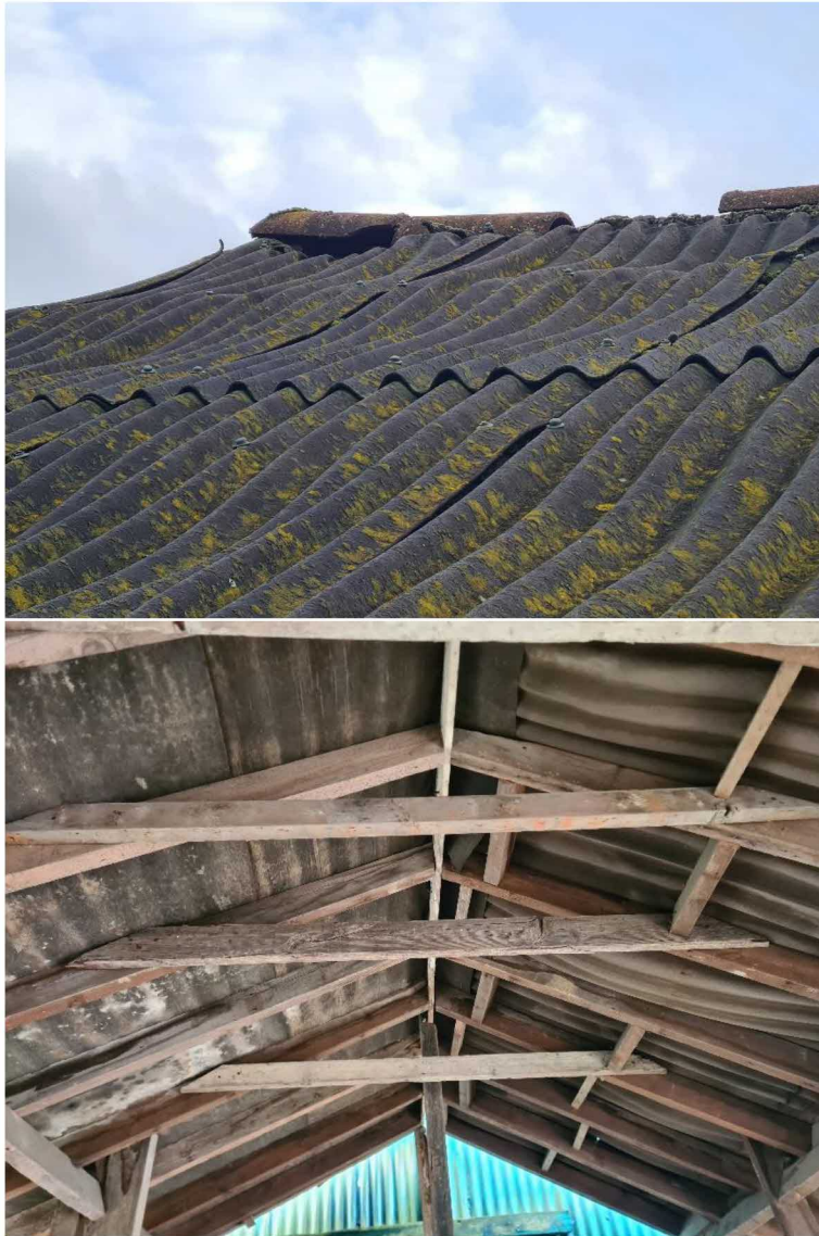
Figure 13: Corrugated roofing felt gaps on the western roof slope of B1a.
