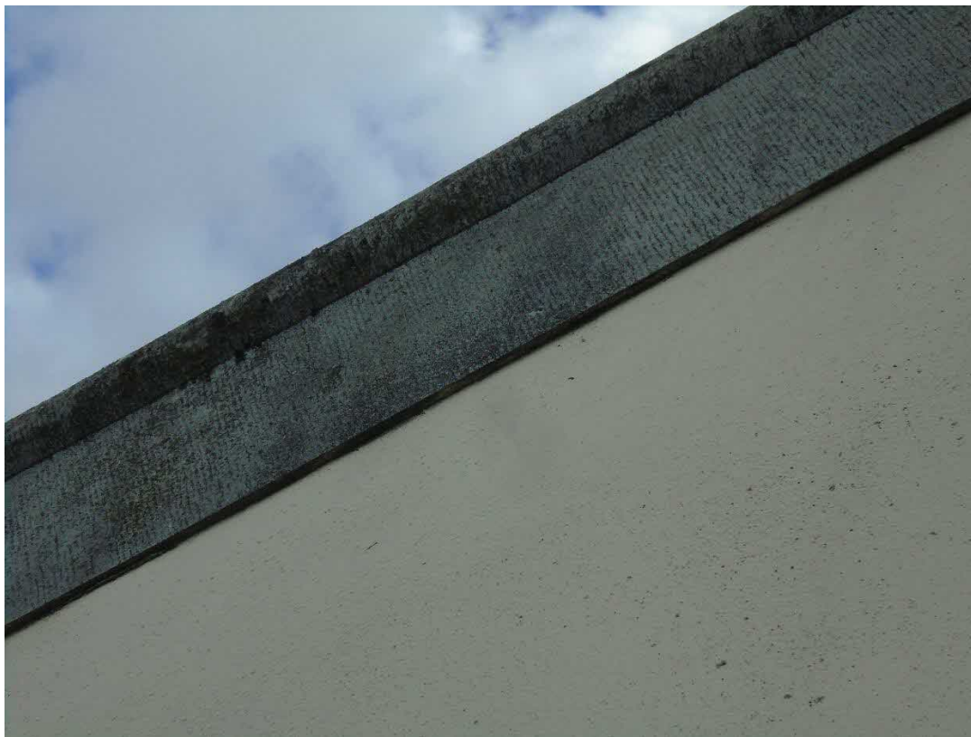
Roof flashing gap less than 5mm wide, with no bat evidence and no potential for bat entry
