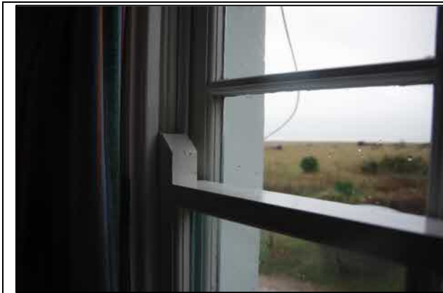
Example of crude and incorrect detailing at the meeting rail of sliding sash
