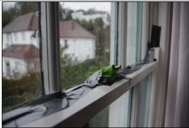
Extremely draughty window taped up
