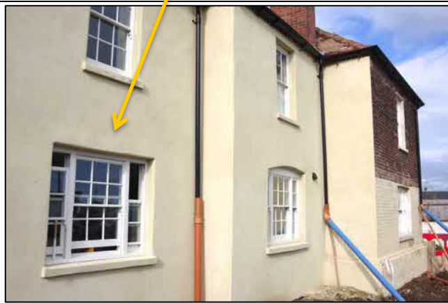
Arrowed yellow line is pointing at the during and after alterations and repairs
