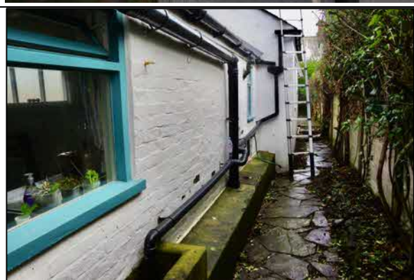
Combined foul and rainwater being run in the same drains at the side of the extensions
