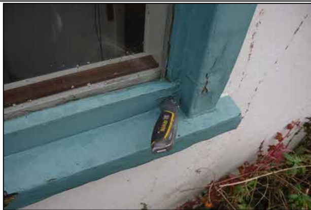
Decaying timber at the second extension, at the street scene
